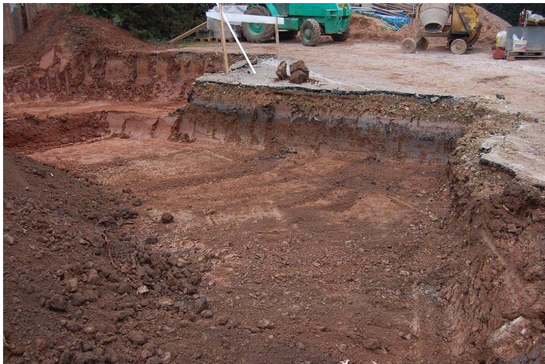
Plate 4: The northern part of the excavated area. Deposit 203 can be seen in the foreground.
