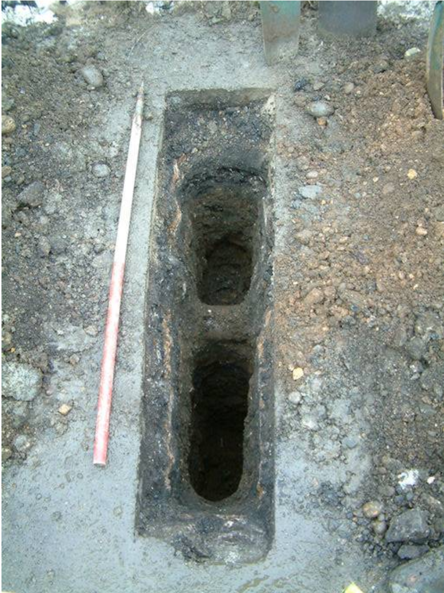
Plate 2, Trench 1, showing tarmac pavement and deposits beneath, truncated by modern services, view north
