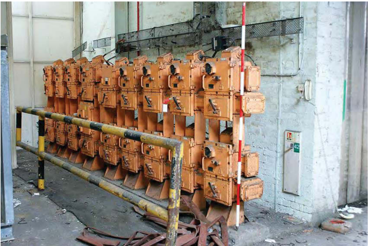
Plate 26: Building B, interior bank of control boxes
