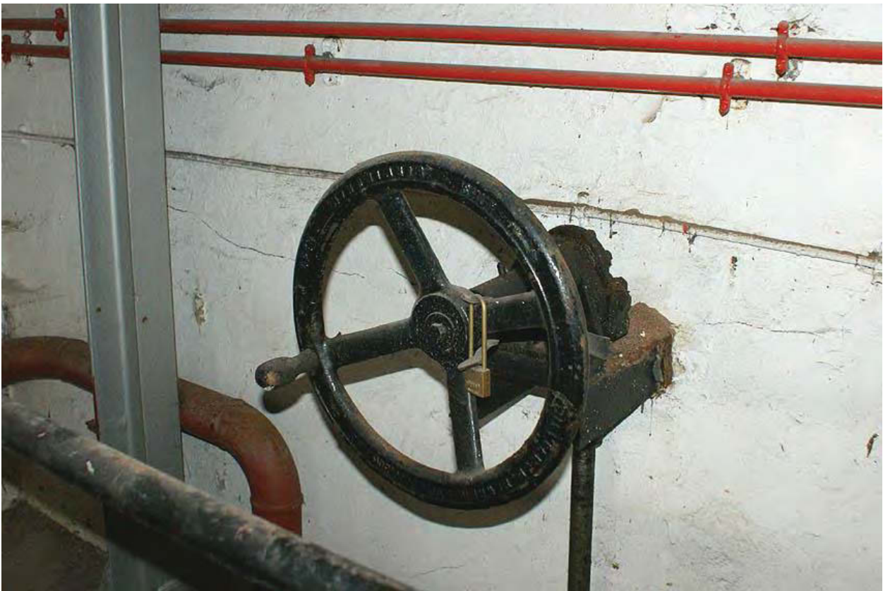
Plate 16: One of old valves in Building A
