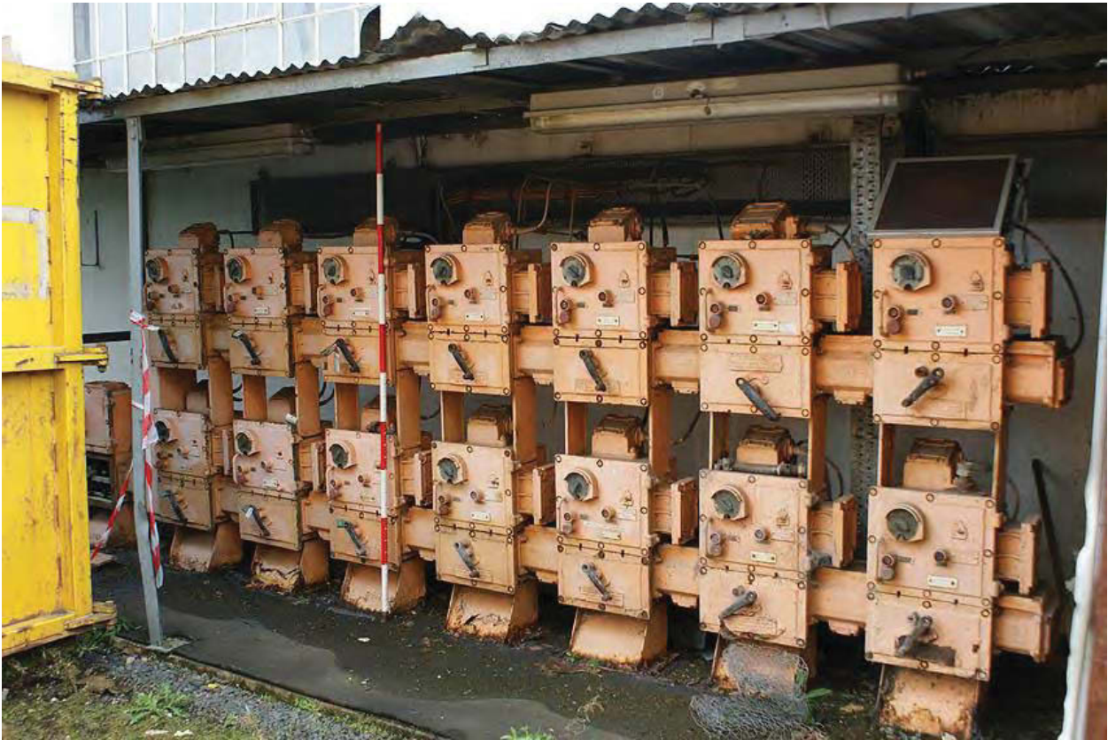
Plate 25: Building B, exterior bank of control boxes
