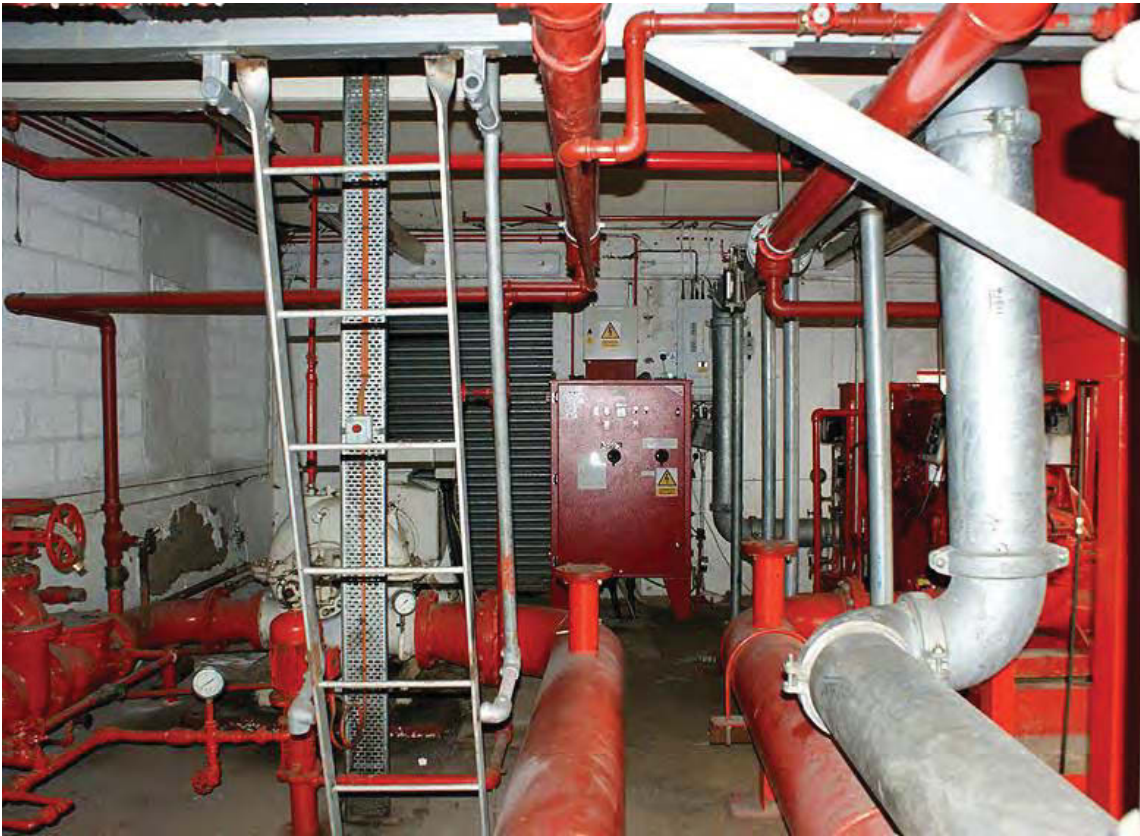
Plate 15: Interior of Building A, showing pipes
