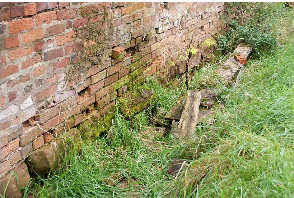
Plate 4: Reused sandstone blocks at the base of northern wall of Building 1, from the north east
