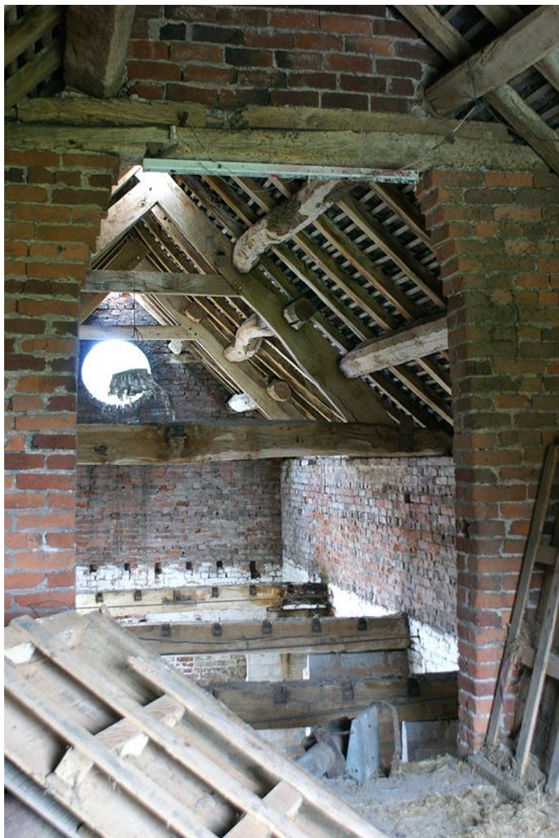
Plate 6: First floor of Building 1 showing trusses and purlin supported by brick division
