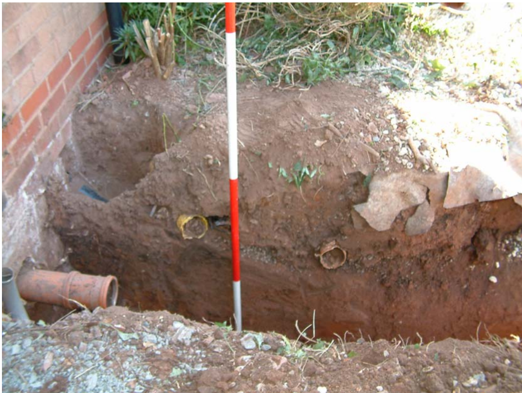
Plate 2: south trench, sample section with modern service ducts and pipes, view south
