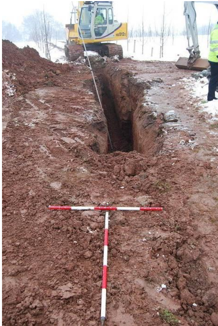
Plate 7, The Service Trench, at the site of the second man hole, facing north
