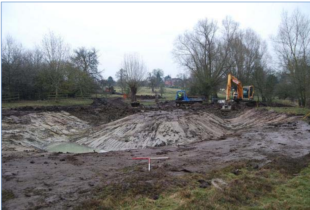
Plate 2 General view of fish refuge 1 at Lower Norchard Farm under excavation, view southeast
