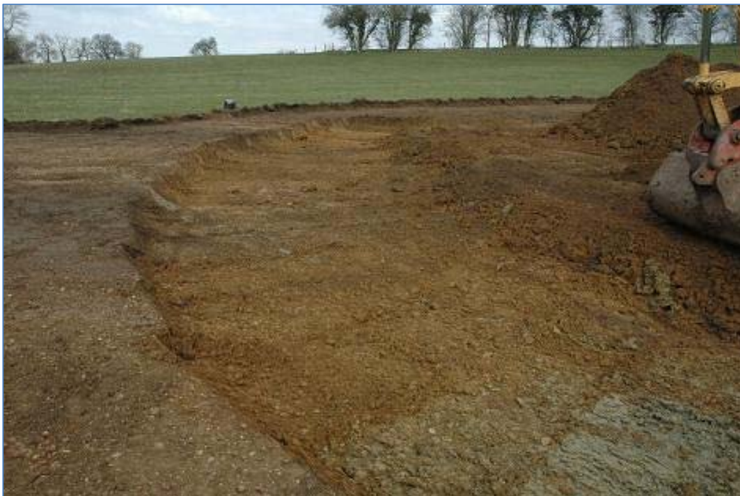
Plate 6 Example of natural river gravels under the furrows and subsoil. View north
