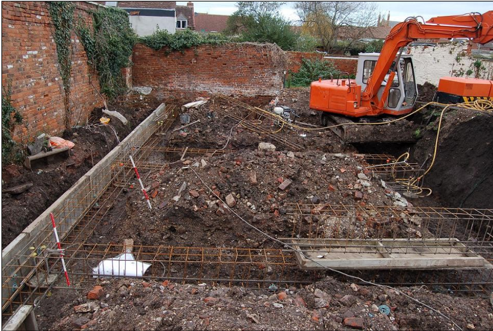
Plate 3: General view of foundation trenches in north end of site, view north
