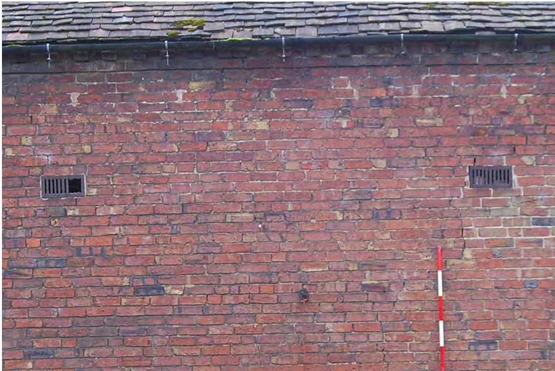
Plate 7: Cast iron 'hit and miss' ventilators, as seen in the north east elevation of Building 3
