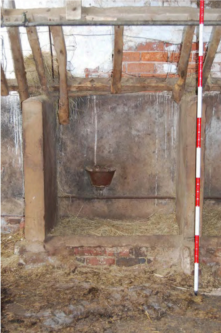
Plate 46: Detail of the feeding trough within Building 11, showing the water system with iron bowls
