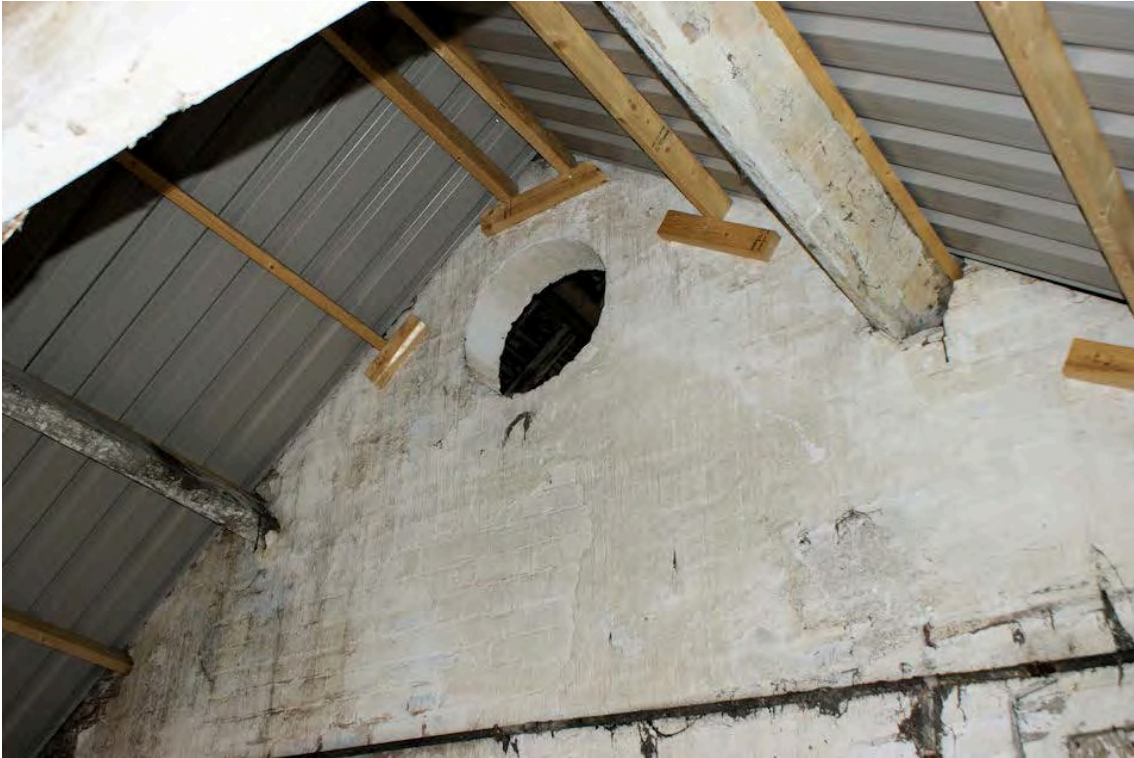
Plate 28: View of the pitching eye in the apex of the south east gable, Building 9
