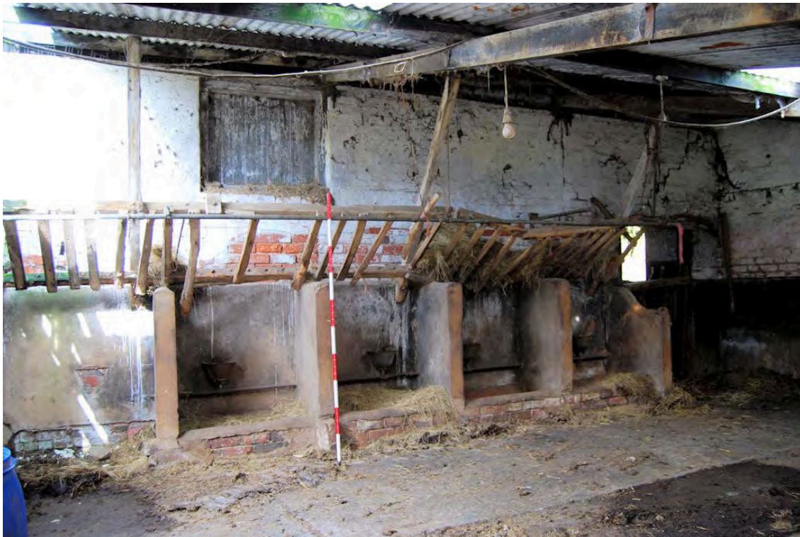
Plate 45: Building 11, brick feeding troughs with ceramic tile lining and concrete covered divisions
