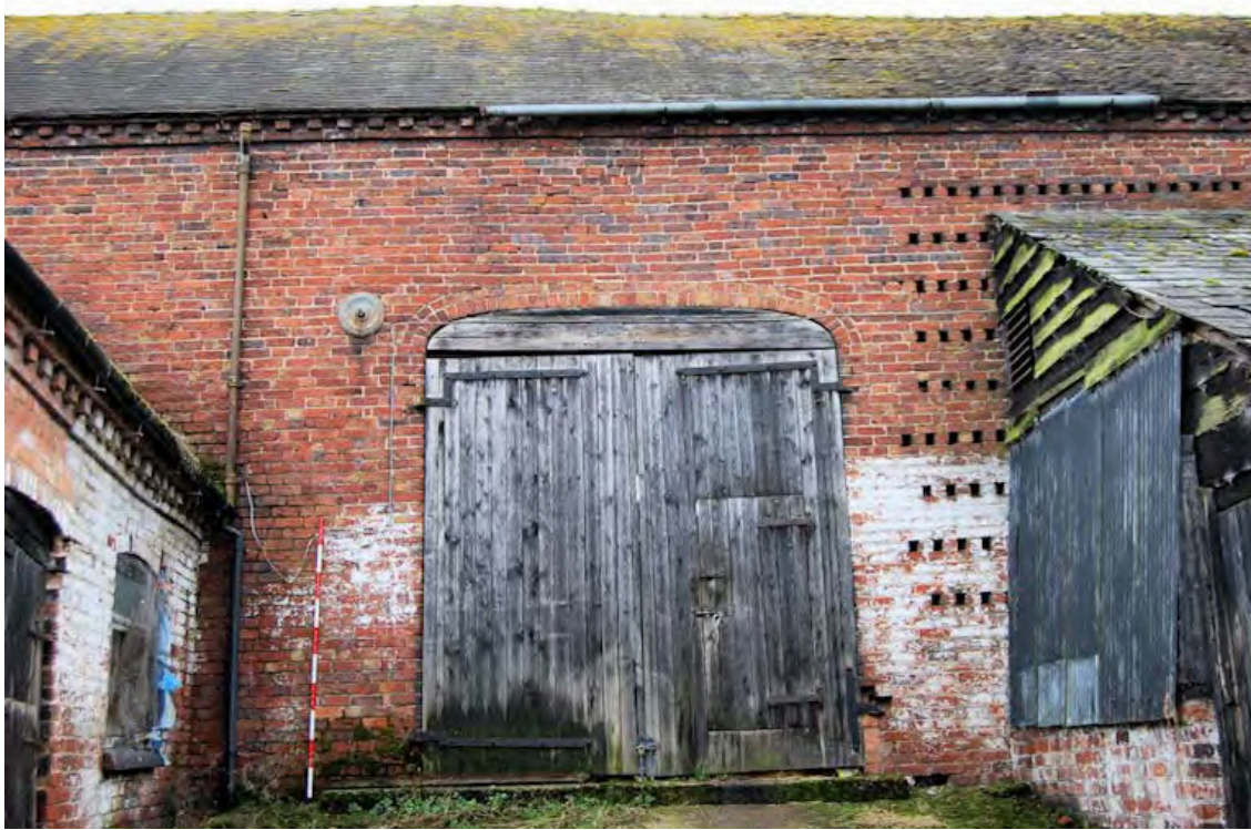
Plate 3: The basket arch of the threshing barn, as seen in the north west elevation, Building 4
