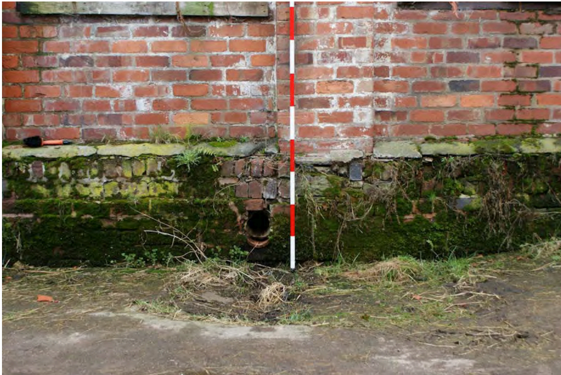
Plate 36: External view of the drain in the north west elevation of Building 5
