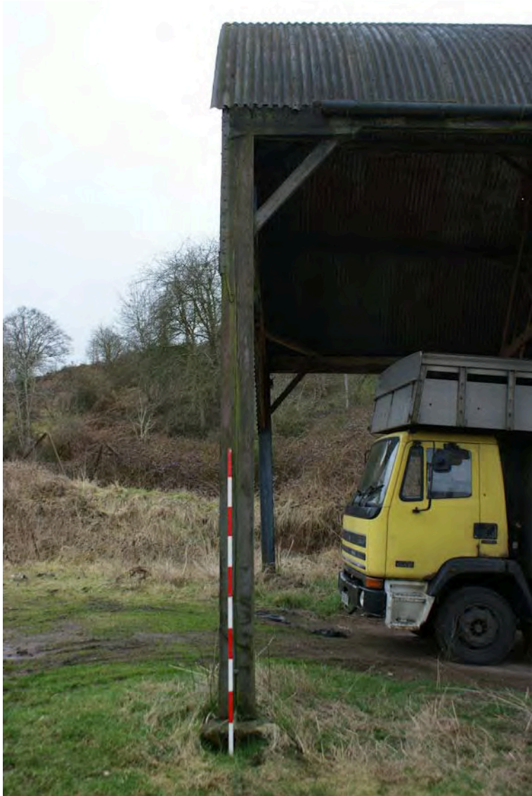
Plate 31: Building 12, an example of a timber post standing on sandstone post pad
