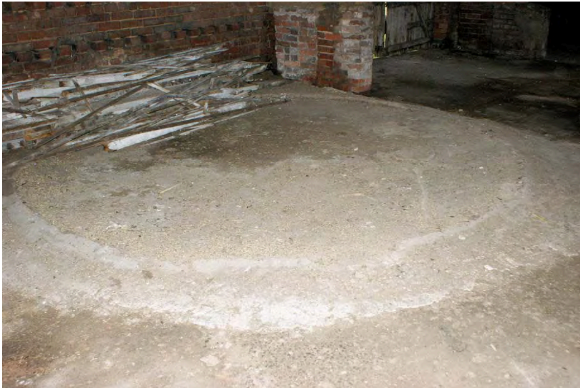
Plate 55: Circular marks on the concrete floor of Building 6
