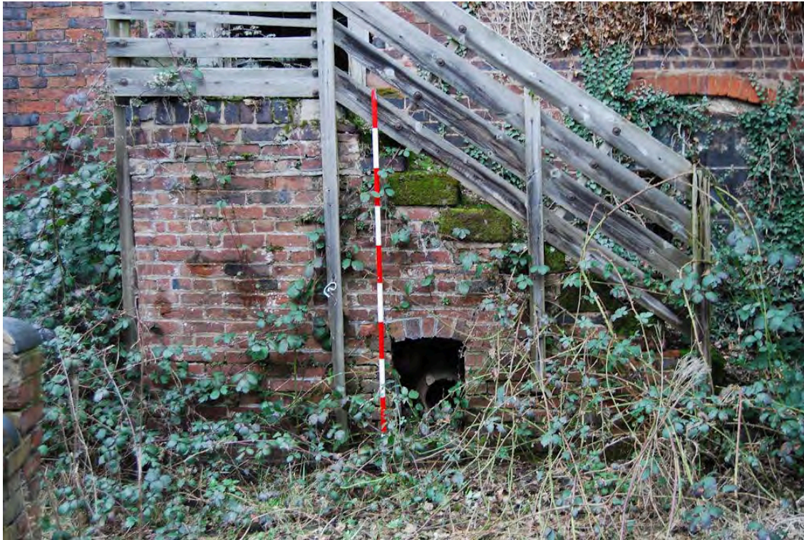
Plate 24: External staircase to provide access to the first floor, including dog kennel
