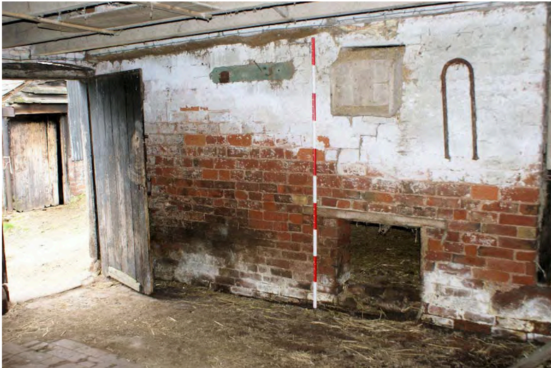
Plate 40: Internal view of mid 19 th century extension to Building 8, showing end of chute, wooden box
