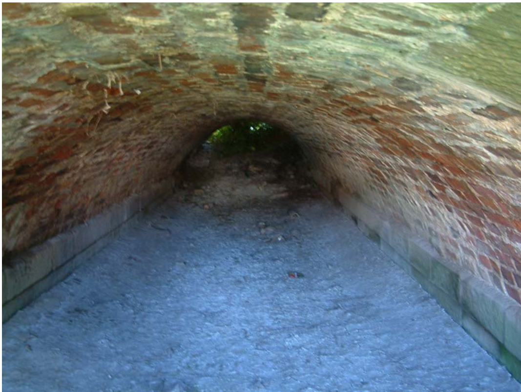
Plate 24 Dumped material at north end of underpass below road.
