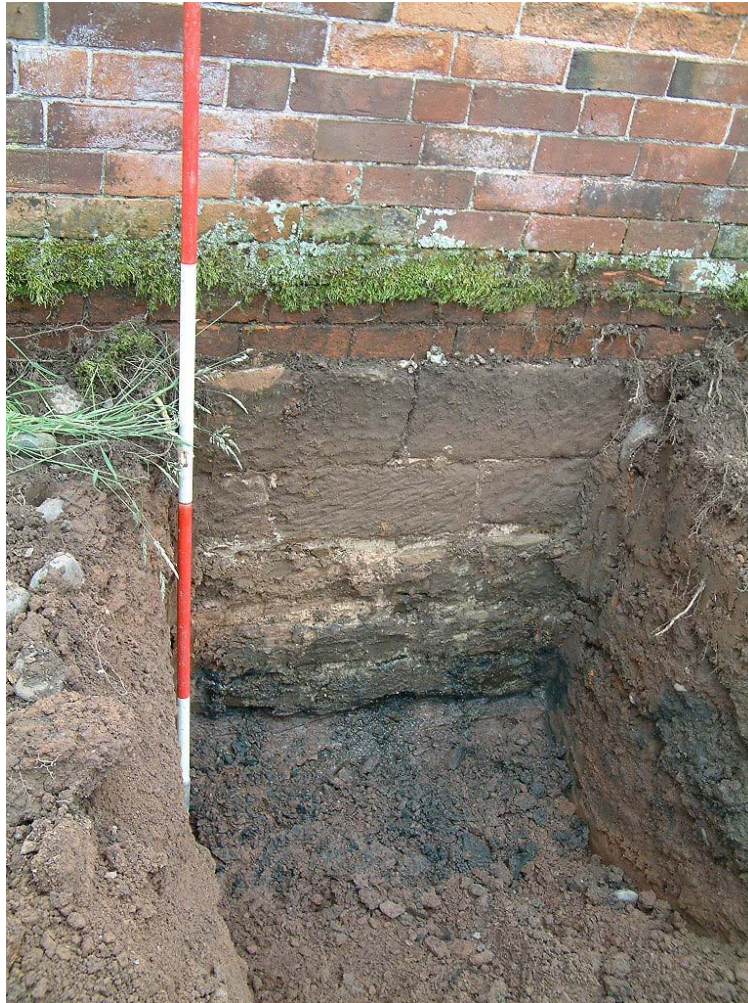
Plate 25 Late 18 th century brick wall with sandstone foundation at Tanwood House, Chaddesley Corbett (Robson-Glyde 2004)
