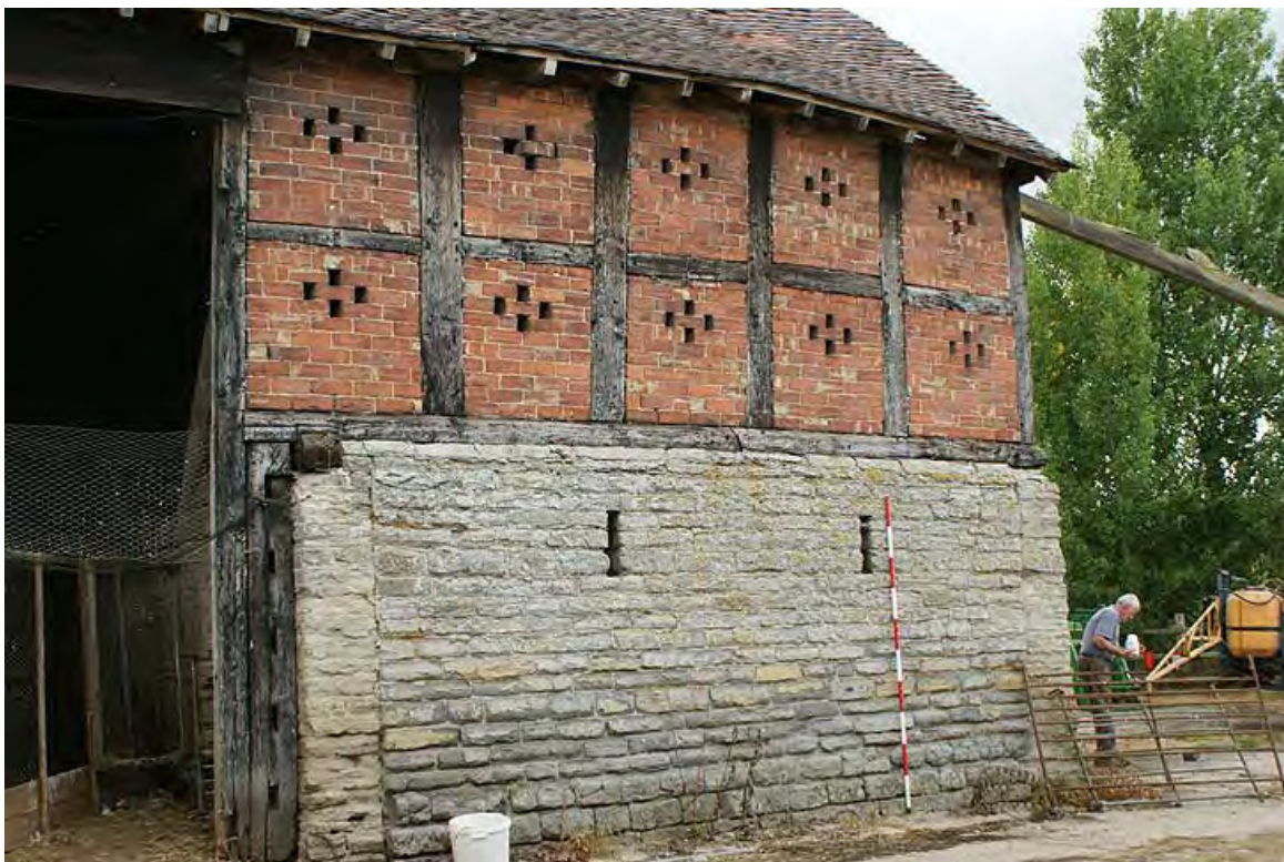
Plate 16: Phase three lias wall and timber frame overlying phase two walls (left and right ground floor)
