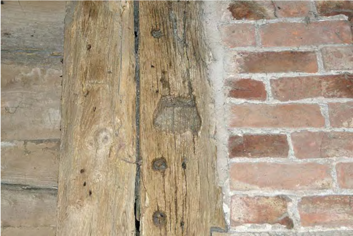
Plate 10: Example of construction notch
