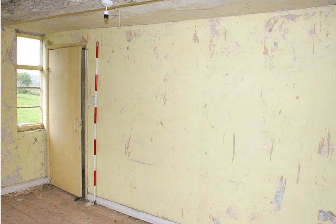
Plate 21: First floor inserted 19 th century partition
