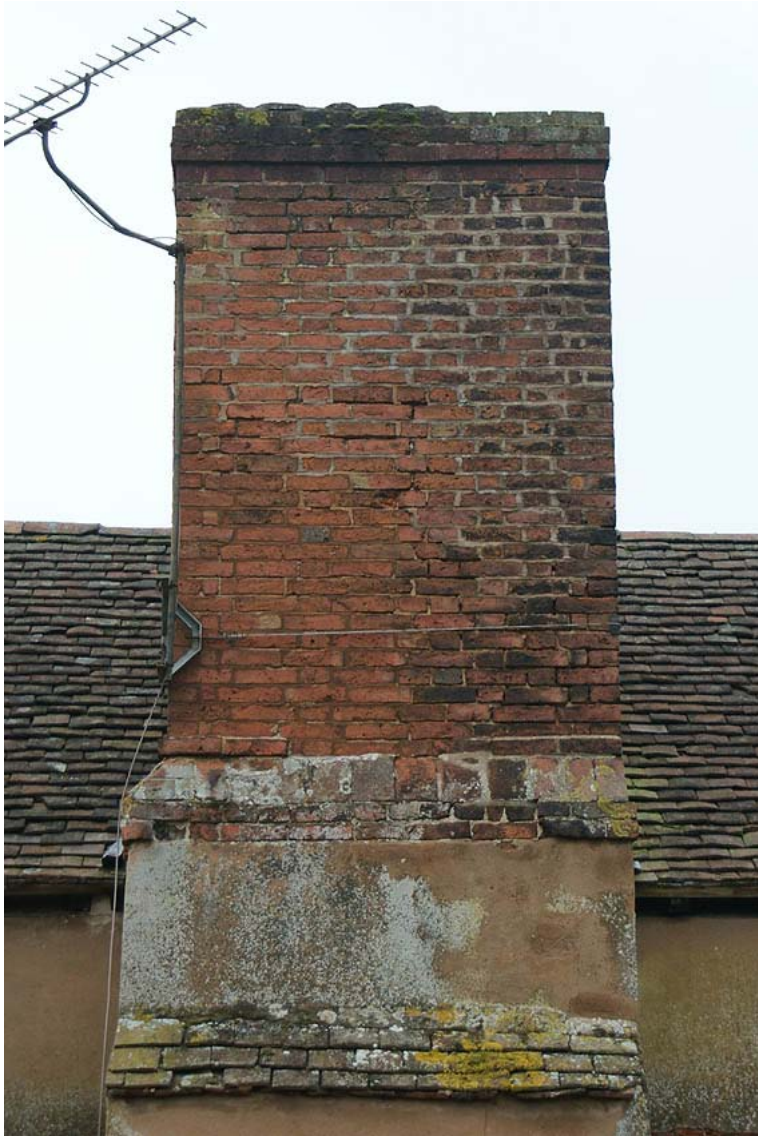
Plate 17: Top of east elevation chimney stack, showing extension on the left (redder bricks)
