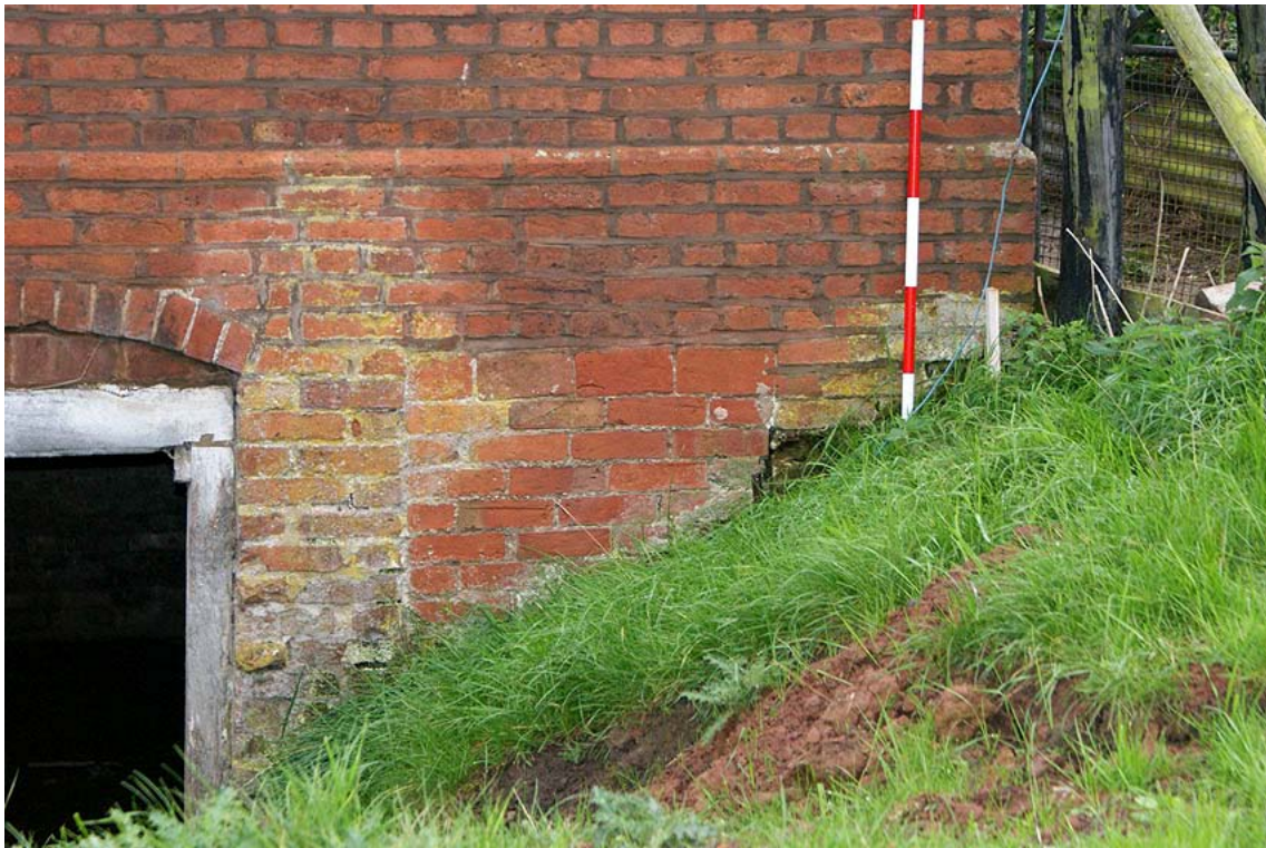
Plate 25: Blocked cellar, stable, window
