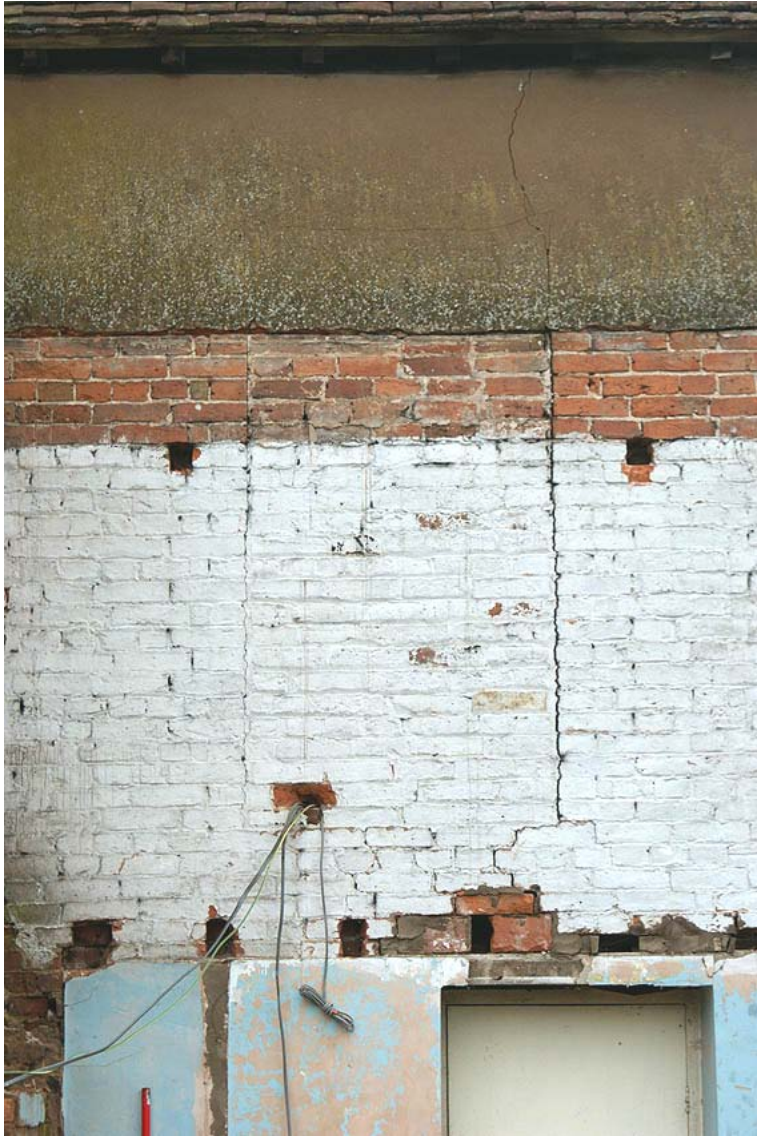
Plate 23: First floor blocked taking-in door
