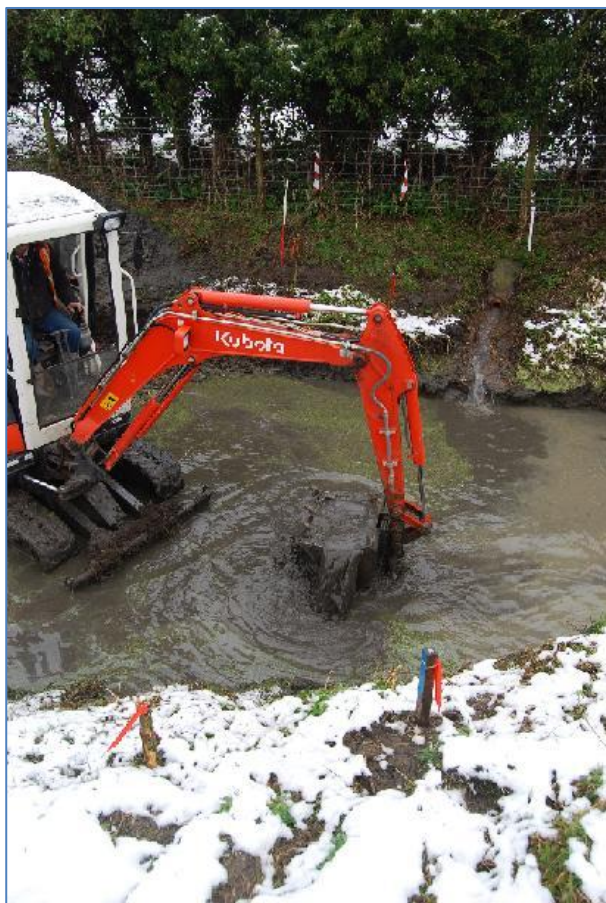
Plate 13 Excavation of a deeper trench between the posts at the centre of the pond, view north
