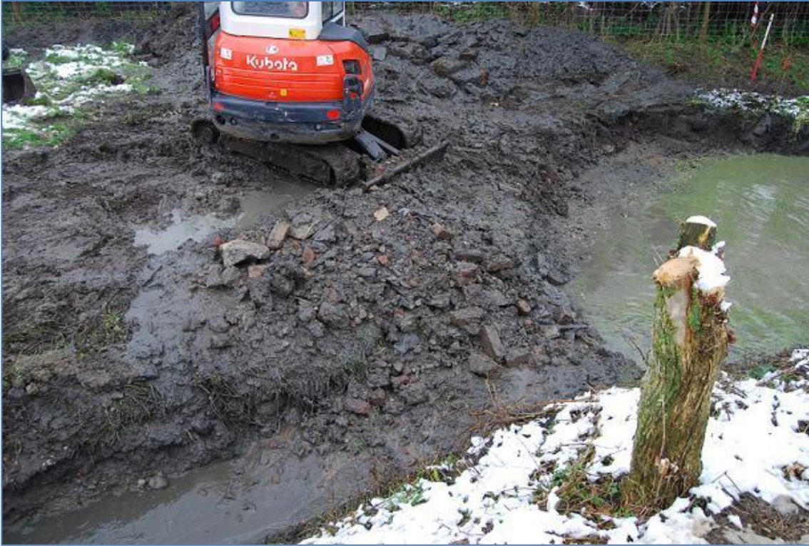
Plate 14 Some of the brick rubble and clay used to block the drainage ditch from the pond, view north
