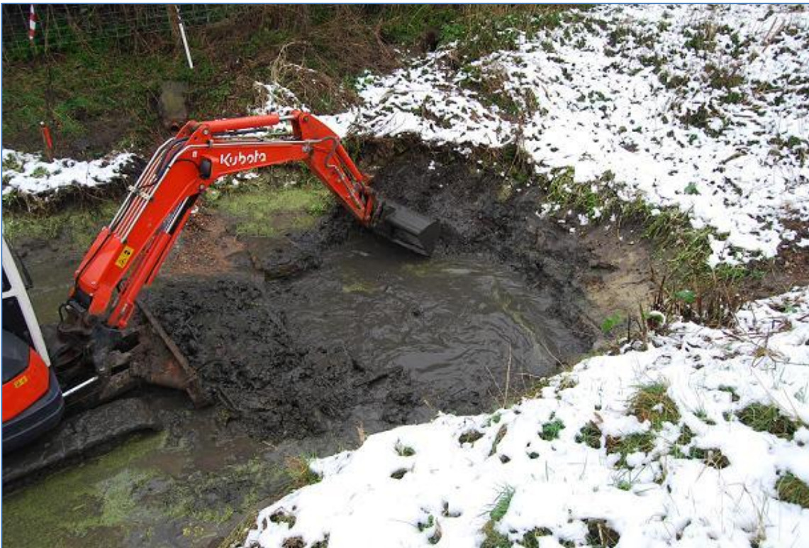
Plate 11 Removing the silt and dumped material from the base of the pond, view north-east
