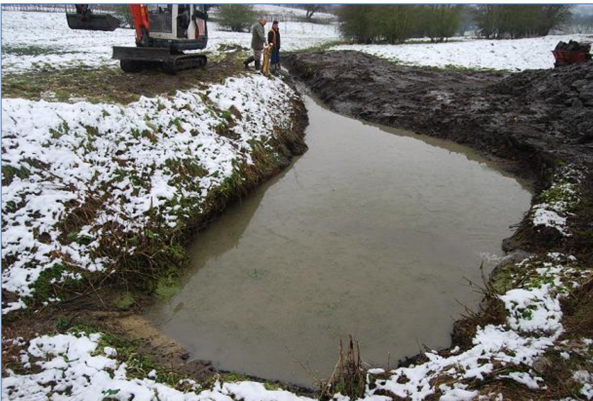
Plate 15 The pond after de-silting works have completed, another wall is visible on the south side, view southwest
