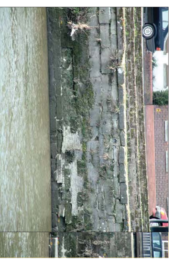
6: Extensively repaired 17th century wall with mooring rings and putlogs
