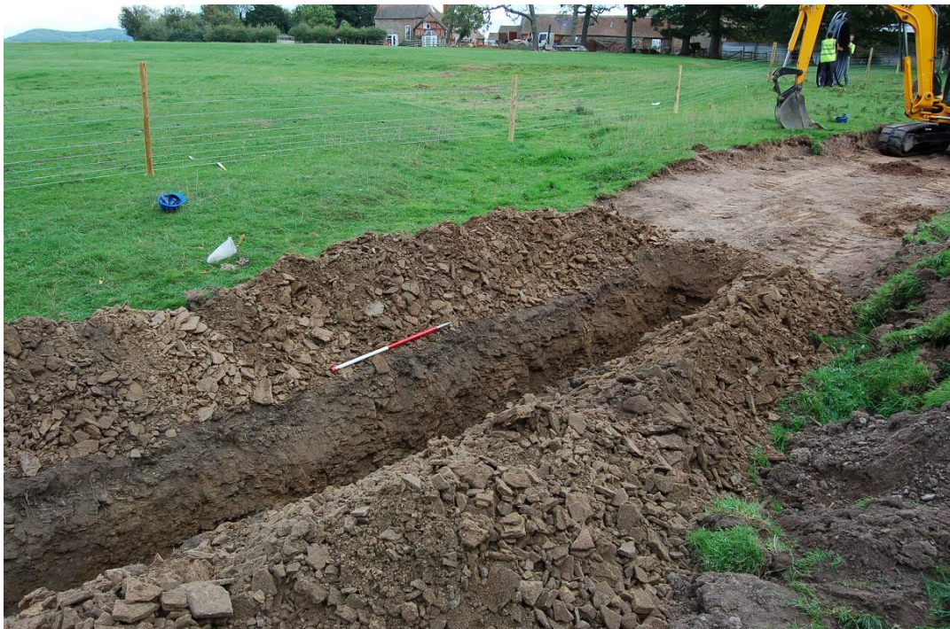
Plate 2: Excavated section of pipe trench through Hollow Way 103. The dark deposit 104 filling the Hollow way is visible in the top of the trench.
