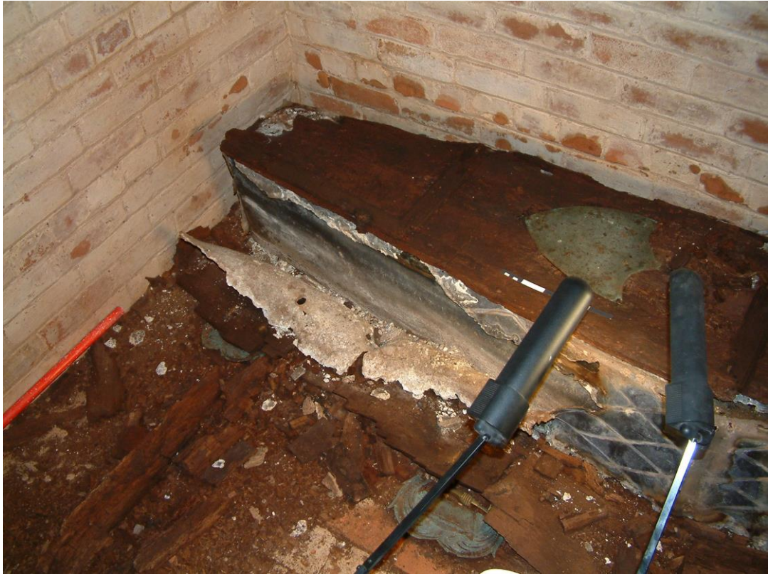
Plate 4: Decay of coffin caused by damp vault conditions (Facing north)
