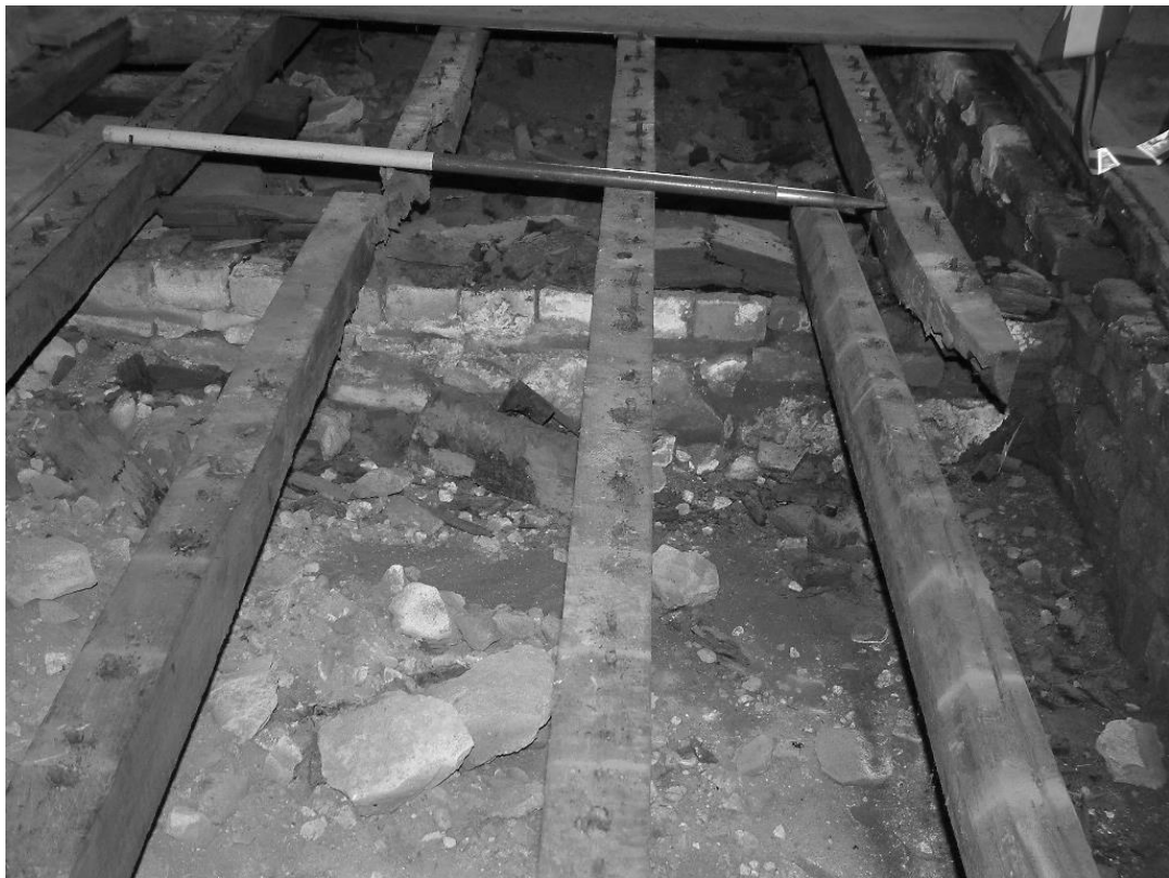
Plate 1: Decayed main bearer supported by brick work (Facing north)
