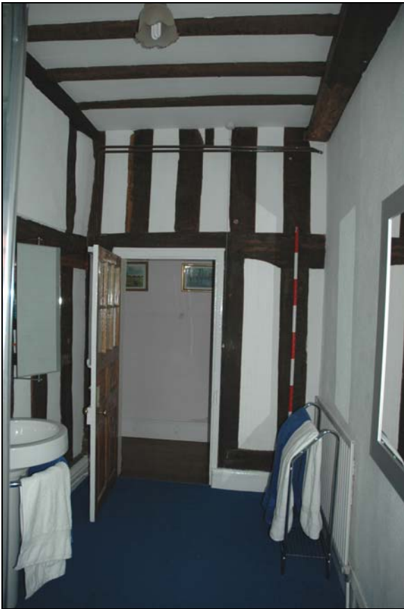
Figure 10: Former doorway now incorporated into the current bathroom of the phase 3 building.
