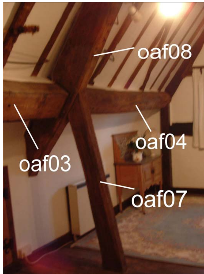
Figure 1: Second floor east room, looking east, showing some of the timbers sampled for dendrochronology
