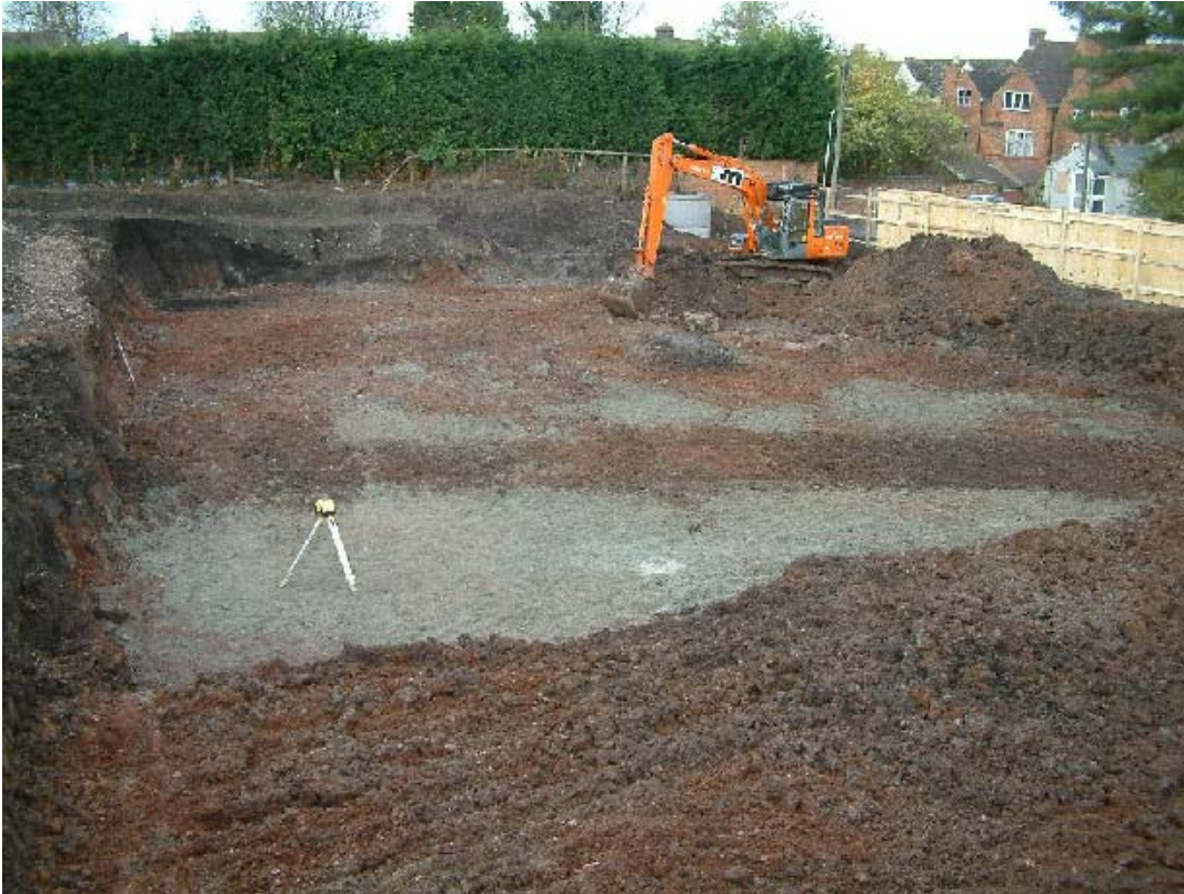
Plate 14: Site after contractor machining. Note base of the large ditch still visible across the site
