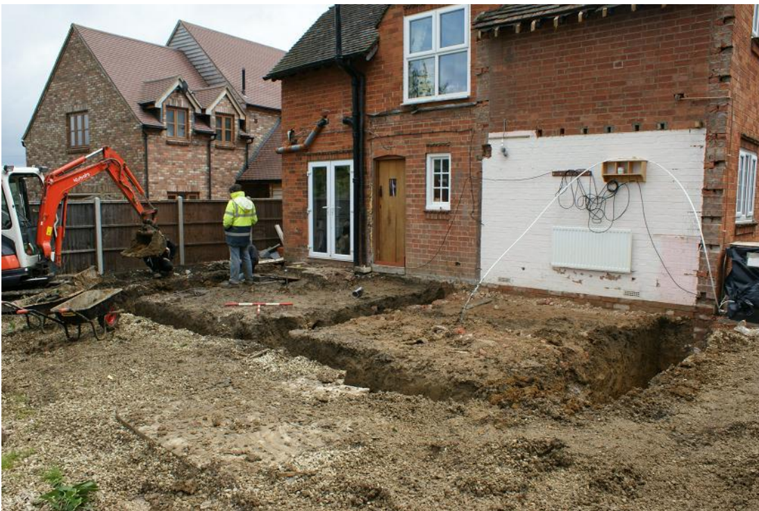
Plate 6 General view east of the site after excavation of all foundation trenches
