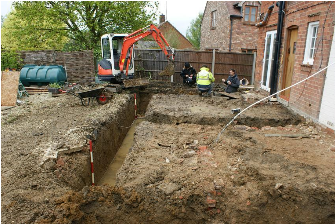
Plate 7 General view north-east of the site after excavation of all foundation trenches
