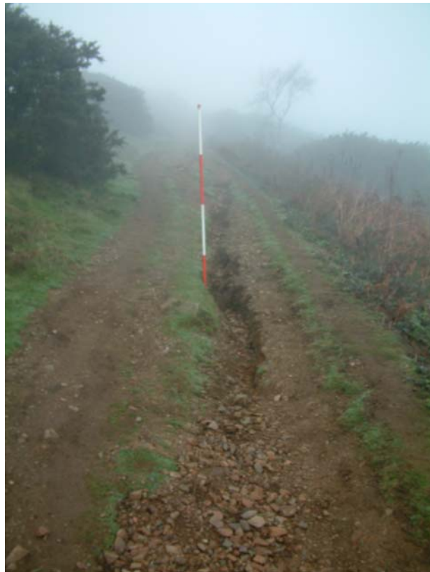
Plate 10: Unit 21, view north of water erosion to path on bank, gorse on ridge and bracken in ditch on Summer Hill (Photo 187).
