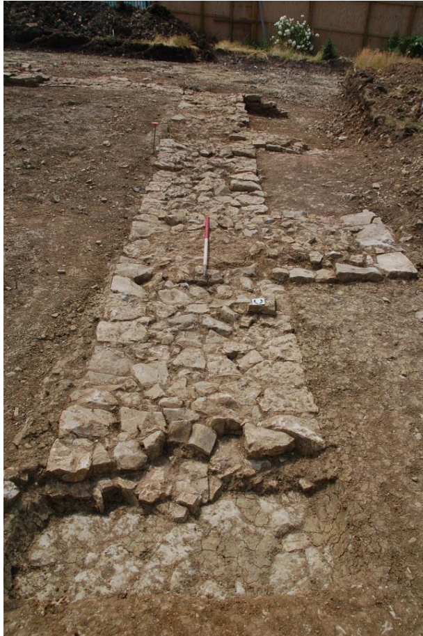
Plate 5: Detail of the western gable end of the tithe barn foundations, facing south, scale 1m
