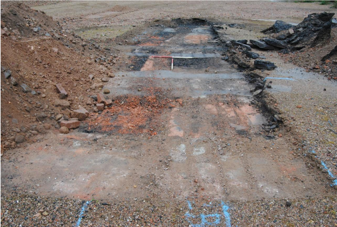
Plate 4. Trench 2 showing the reinforced concrete slabs below the tarmac/rubble ground surface. Photo looking west
