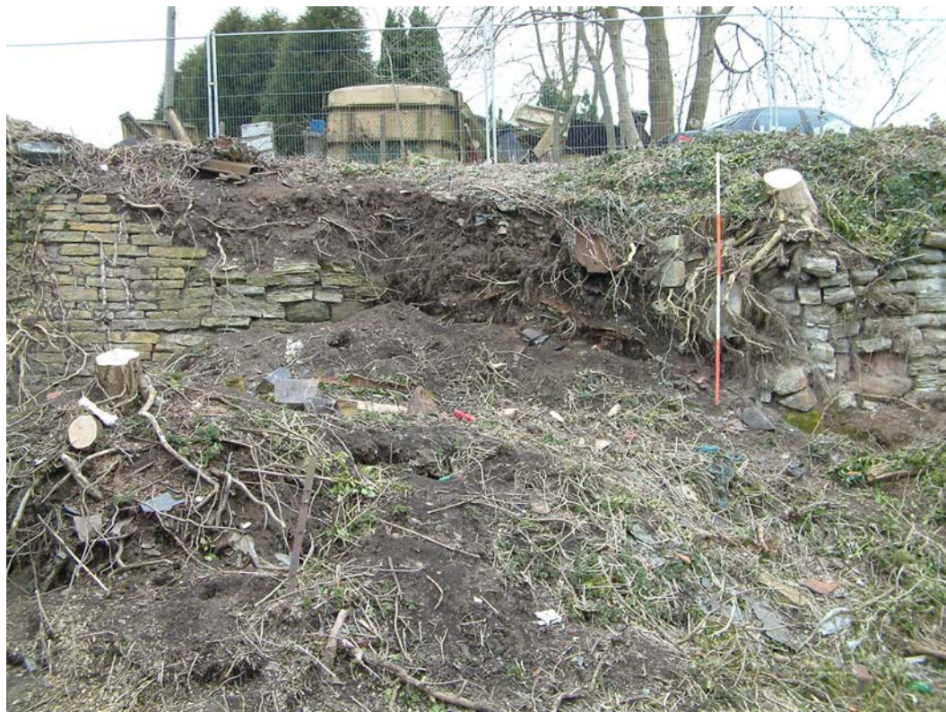
32. Kiln bank façade collapsed between Kilns 1 & 2 and 3-5, view south-east
