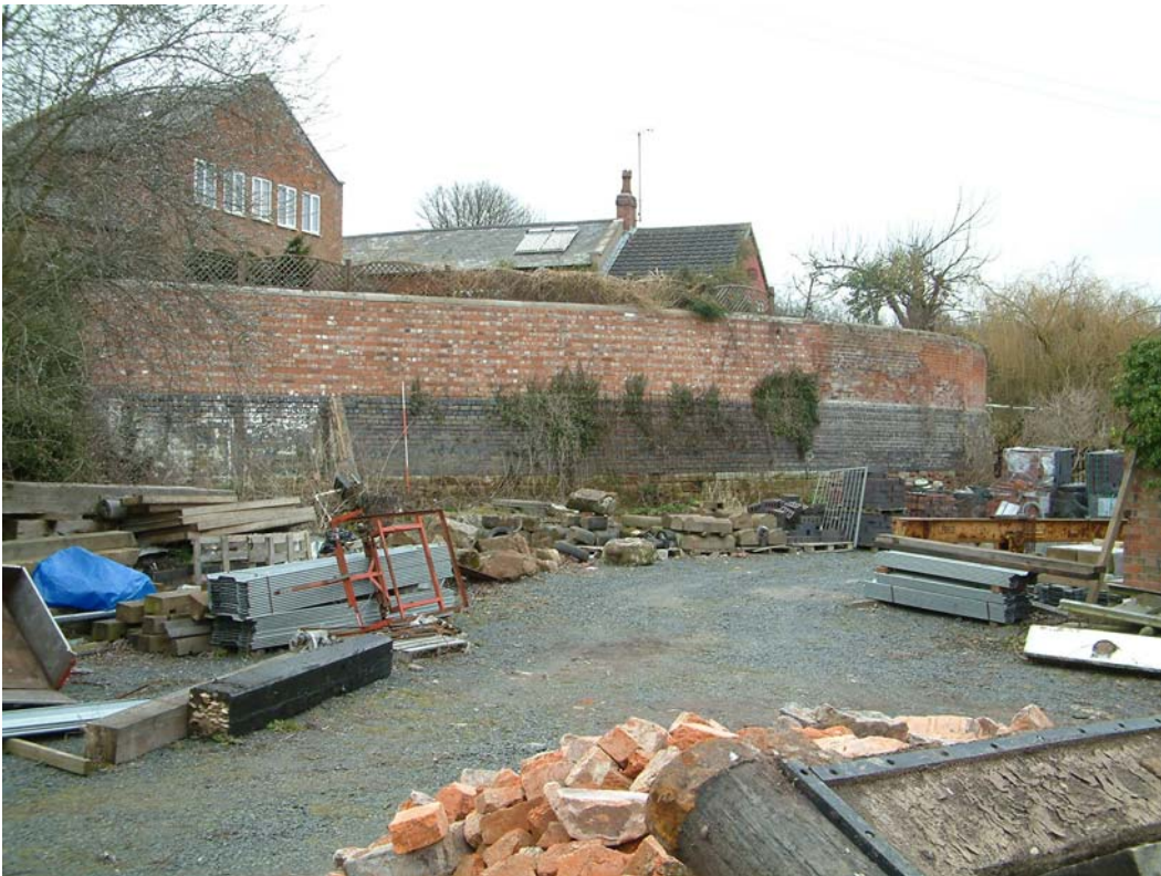
8. Plymcot retaining wall and site of former stables and closet, view east-south-east
