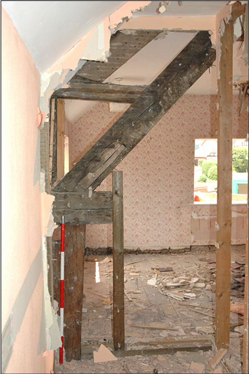
Plate 10: Room 21, cut off tie beam extending beyond length of principal rafter
