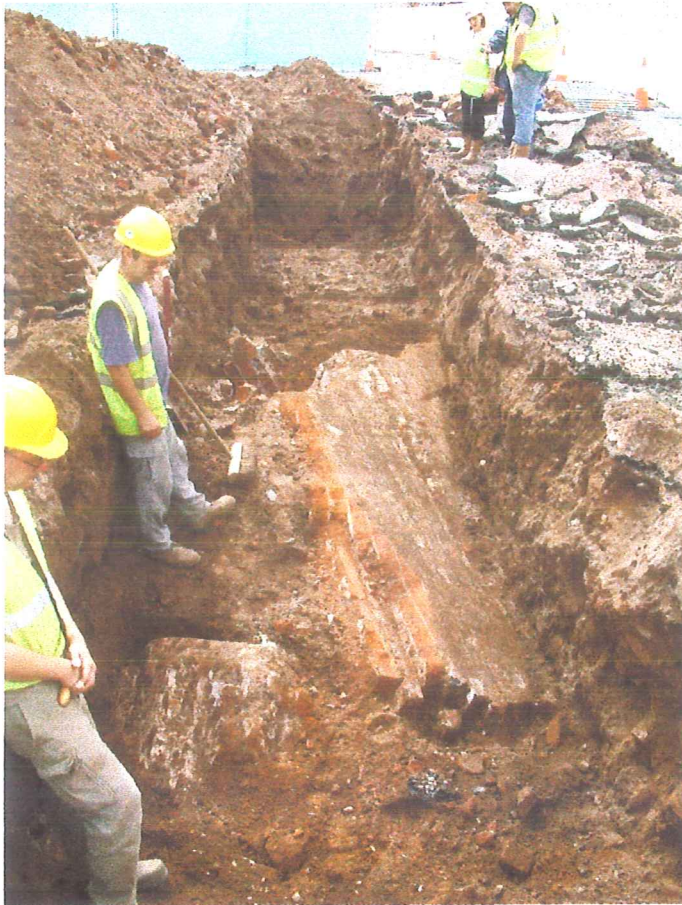
Plate 1, Collapsed wall in Trench 1
