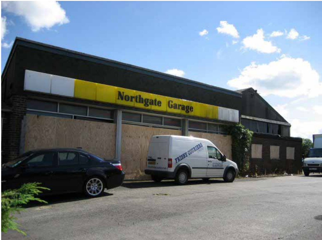
Plate 27. The Northgate Garage, North Gate. A C20th brick building, identified for demolition in the planning application: the new relief road will run through here (see Fig 4).
