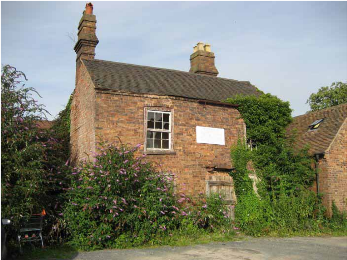
Plate 23. No. 5 Whitburn Street. A 19 th century brick two-storey, three-bay house, now uninhabited and derelict. This house was originally accessed by a lane between Nos. 4 and 5 Whitburn Street (see Plate 21), which led to a garden in front of the house, shown on Ordnance Survey map of 1884 (see Fig 9). There is some evidence for subsidence on the north side of building, where it stands over the town ditch (see text).
