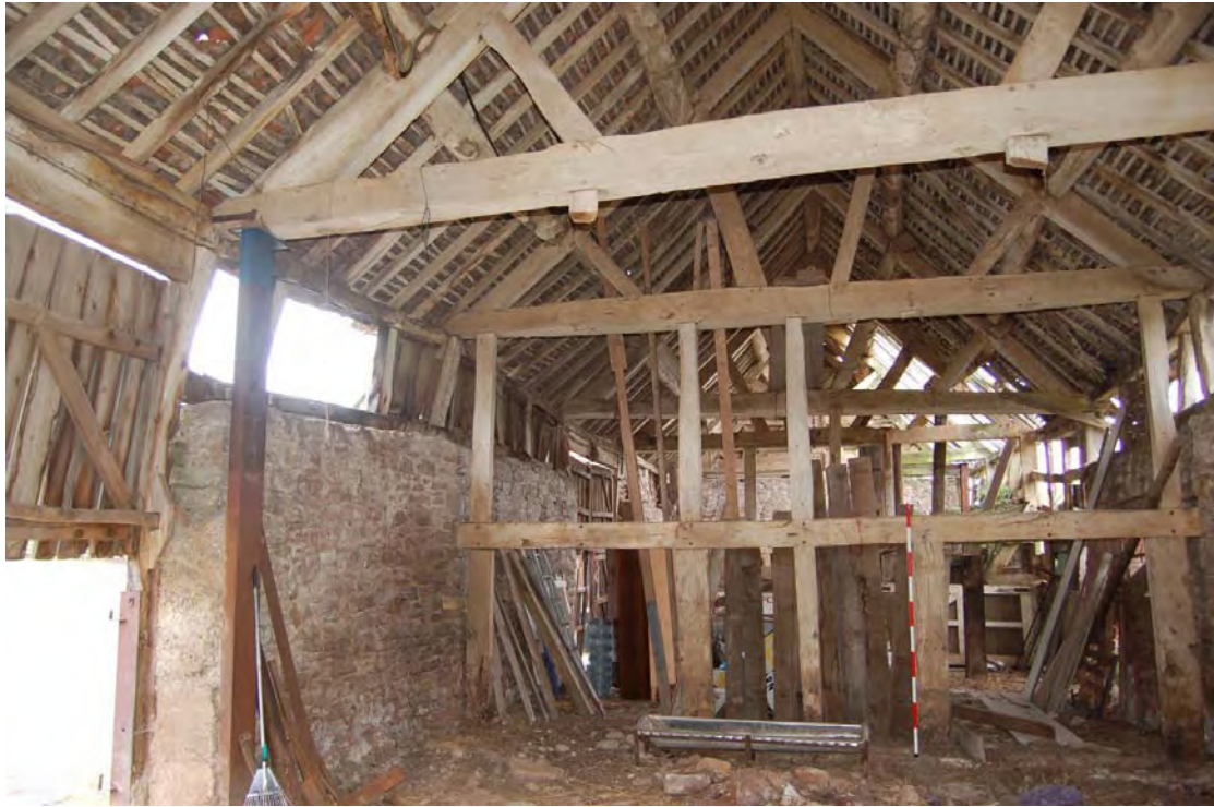
Plate 11: The Barn, evidence of original divisions of barn into bays (see remains of lower timbers below truss in foreground)
