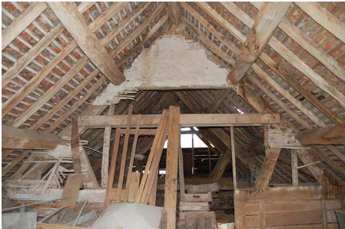
Plate 29: The Stable, west room, upper floor showing remains of plaster on partition.
