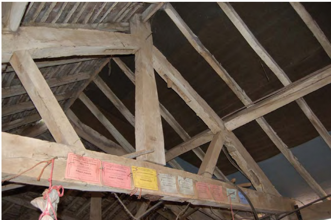
Plate 37: The Animal Shed, Room C, King Post showing example of empty mortices suggesting re-used timbers were included in the construction of the building.
