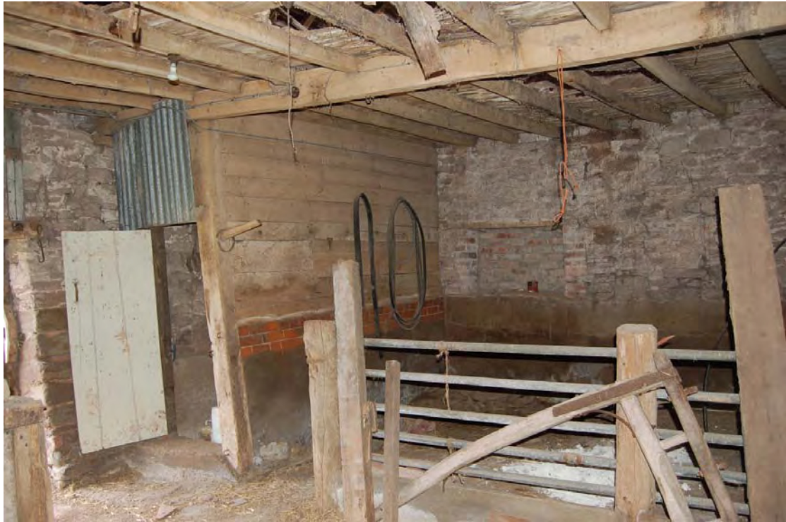
Plate 28: The Stable, east room ground floor showing remaining post of partition and tack room with saddle attached to outside of door jamb.
