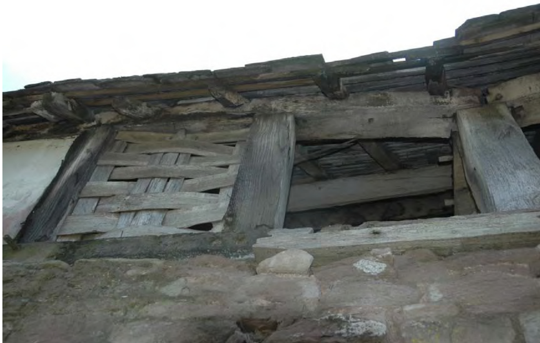
Plate 6: The Barn, detail of square panelling and oak wattle and empty panel showing auger holes where wattle removed.
