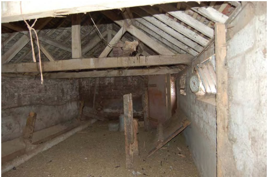
Plate 21: The Animal Shed, Room C, looking south east showing door in the distance and remains of corridor.
