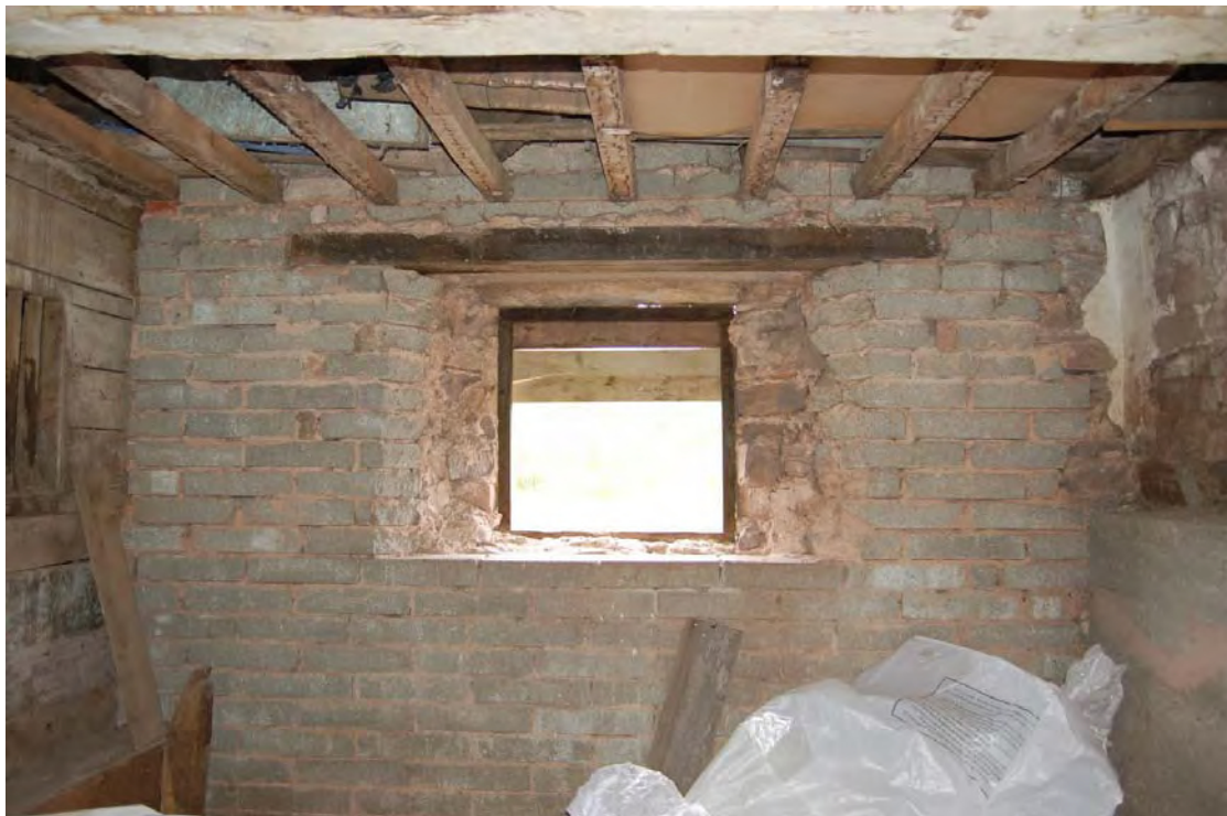
Plate 25: The Stable, west room, ground floor, showing plaster covering red sandstone in corner of western wall and remains of southern wall.
