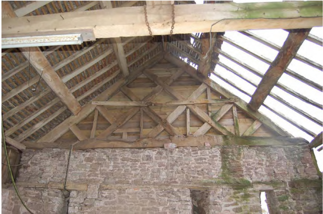
Plate 7: The Barn, east end showing diamond panelling. Auger holes in the panels show that original wattling has been removed.
