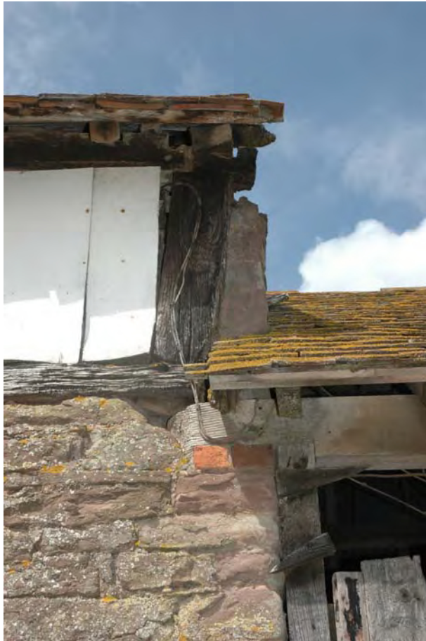
Plate 5: The Barn east end with Animal Shed adjoining, showing square panel with wall plate below and roof plate above.
