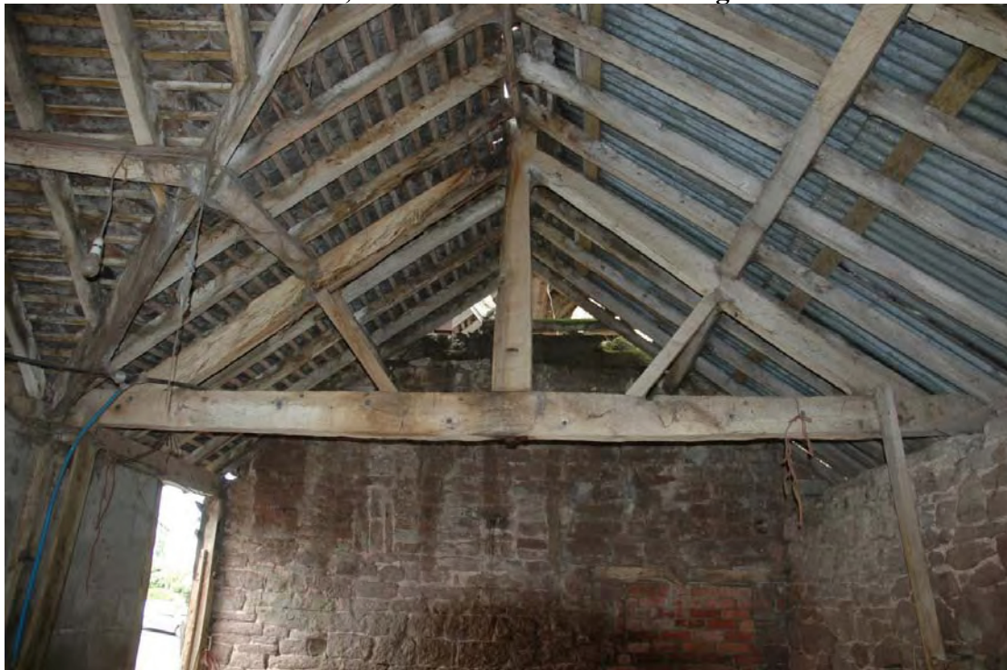
Plate 19: The Animal Shed, Room A, showing exterior of western wall of Barn A and King Post with metal bolt below the tie beam and small slot in Post above where nut inserted.
