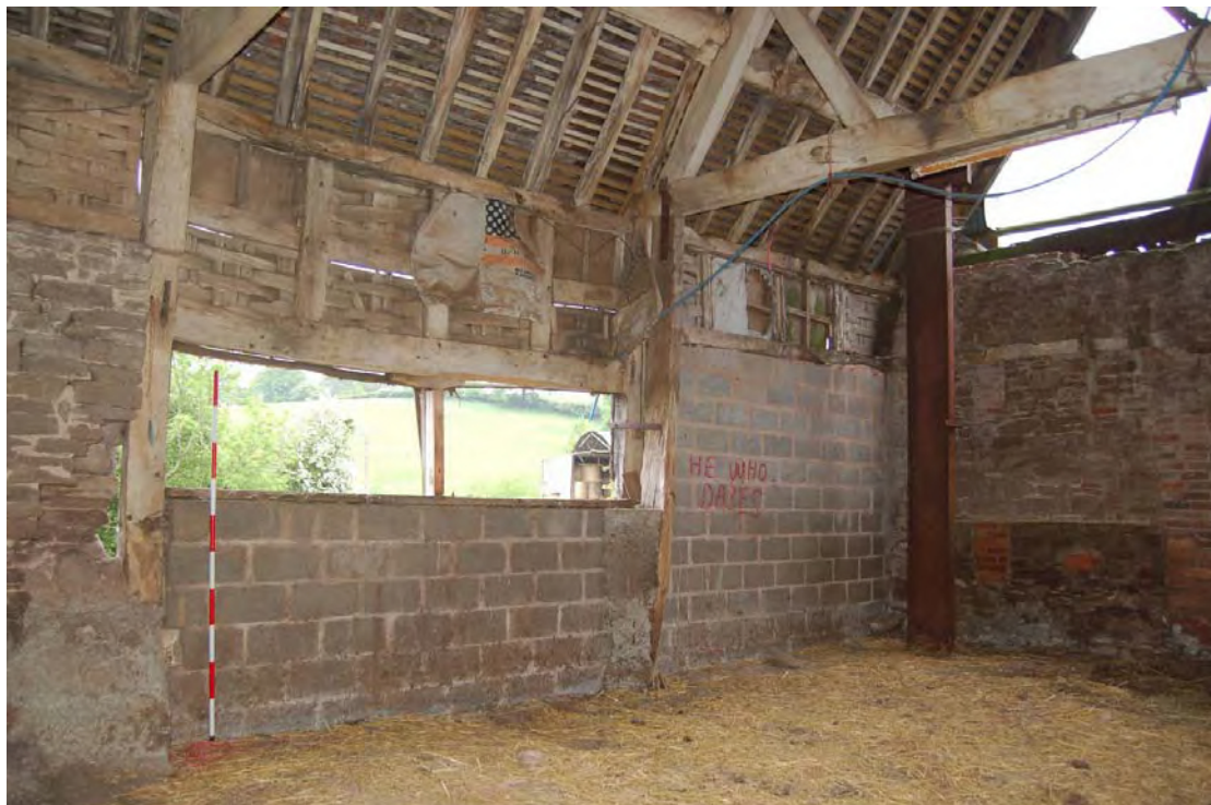
Plate 10: The Barn, north wall showing original panelling within original doorway opposing present south doorway.
