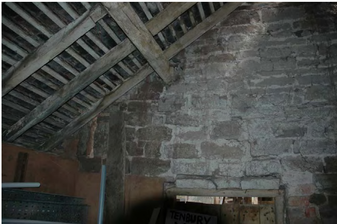
Plate 31: The Barn, exterior of west wall within adjacent farm building with central door of The Barn at bottom of photograph and ventilation hole, now partly obscured by roof, at mid-left of photograph.
