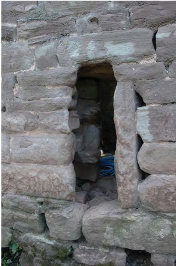
Plate 9: The Barn, showing detail of rectangular ventilation hole as originally built into the wall.
