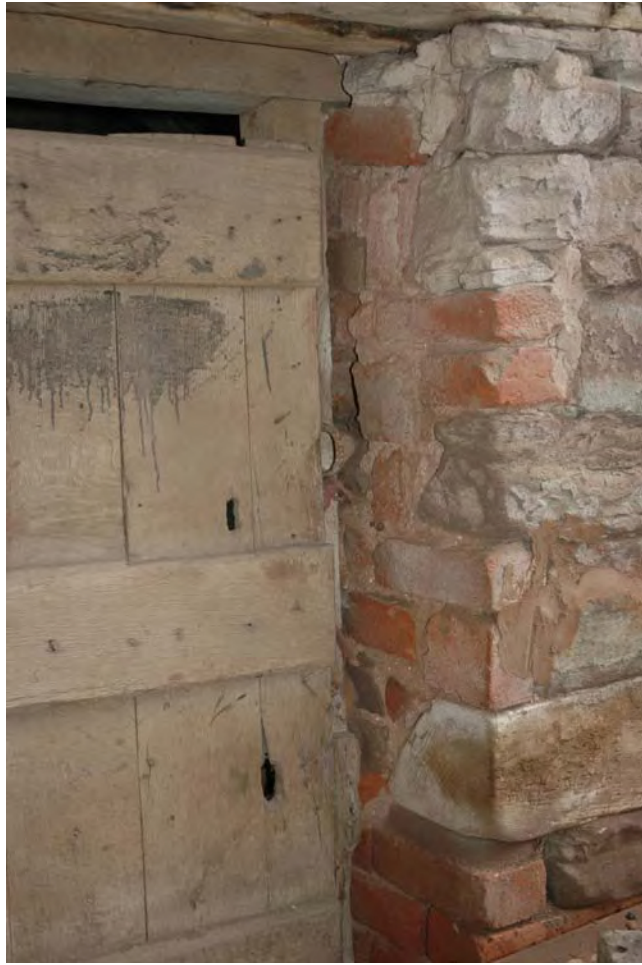
Plate 32: The Barn, detail of central door in west wall from within The Barn.
