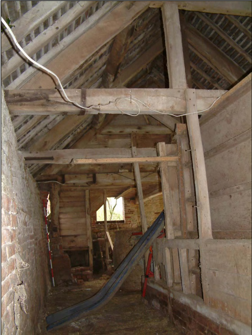
Plate 9: Building 2 looking along feeding passage with remains of brick trough on right
