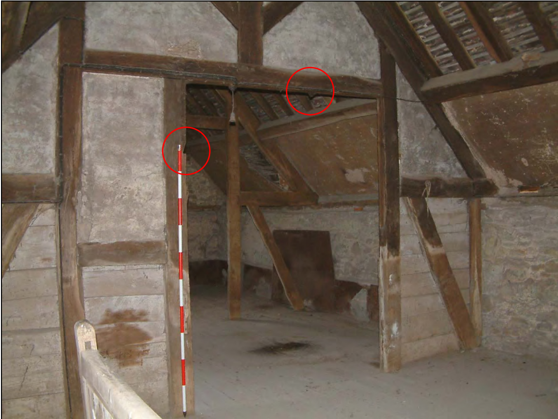
Plate 3: Opening in building 1 timber frame partition with evidence for previous door and window
