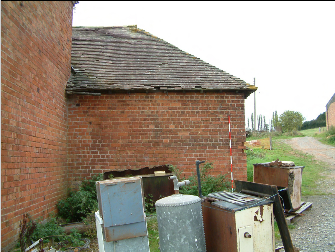
Plate 21: Building 1 early 19 th century boundary wall forming part of late 19 th cart shed
