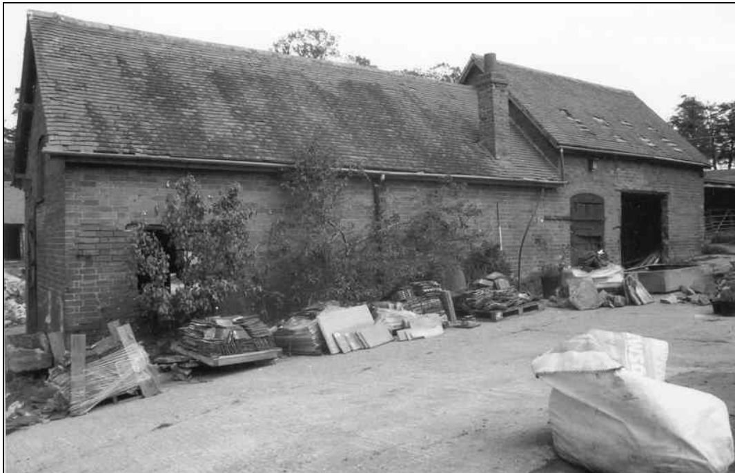
Plate xxii South facing elevation of southern range – wood shed and stores A and B
