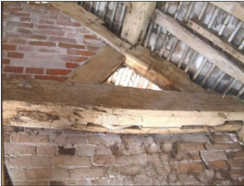
Plate xiv Detail of truss and purlin formation in west elevation of pig cote
