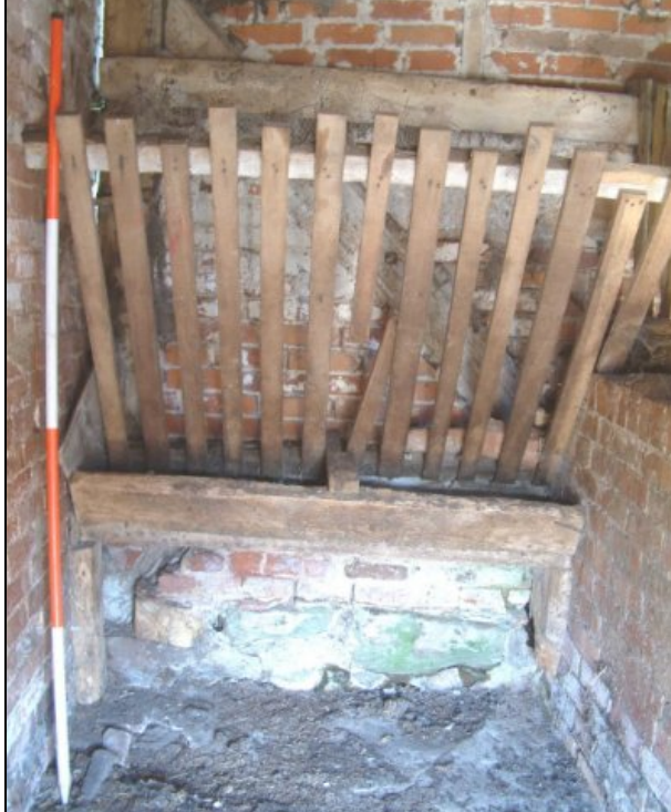
Plate xv Internal south facing elevation in pig cote showing feeding trough and stone footings
