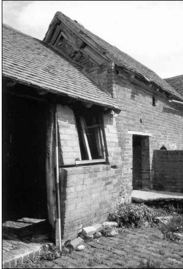
Plate iii Buckling of wall at southern frontage of milking parlour
