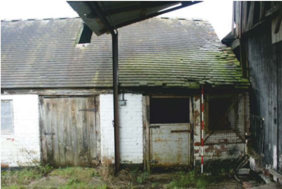
Plate 15 Phase 1 shelter shed with mortice and peg hole above the right hand door, looking north-west
