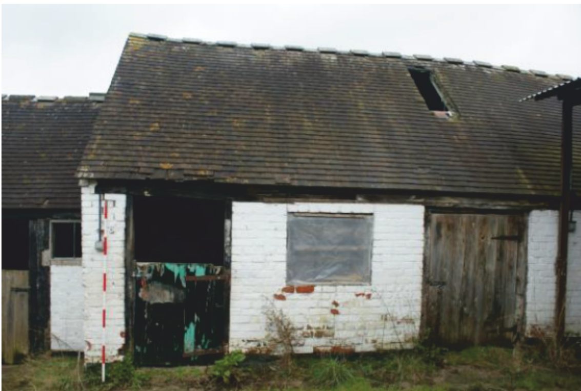
Plate 14 Phase 1 shelter shed with mortice and peg hole above the left hand door, looking north-west
