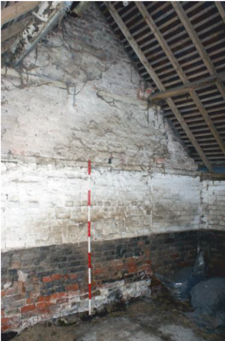
Plate 8 Phase 1 shelter shed with blocked doorway, looking west
