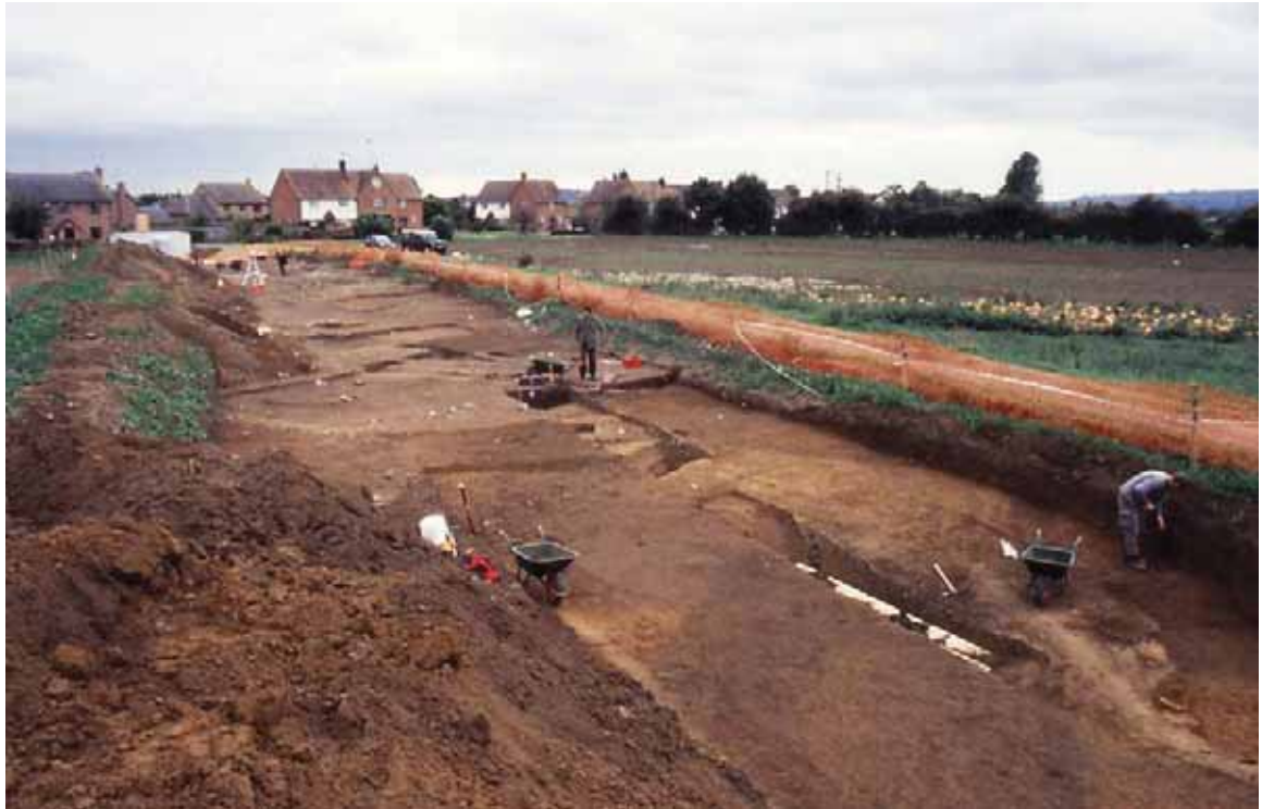
Figure 11. General view looking south across site. Bronze Age ditch (CG1) in lower centre in course of excavation and Roman ditch at right-angles in centre foreground
