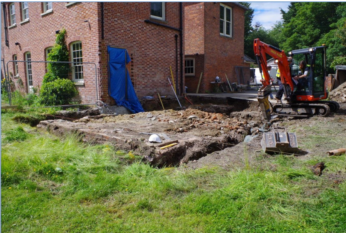
Plate 2 The concrete footings in the northeast corner being broken out during groundworks on Trench 1.
