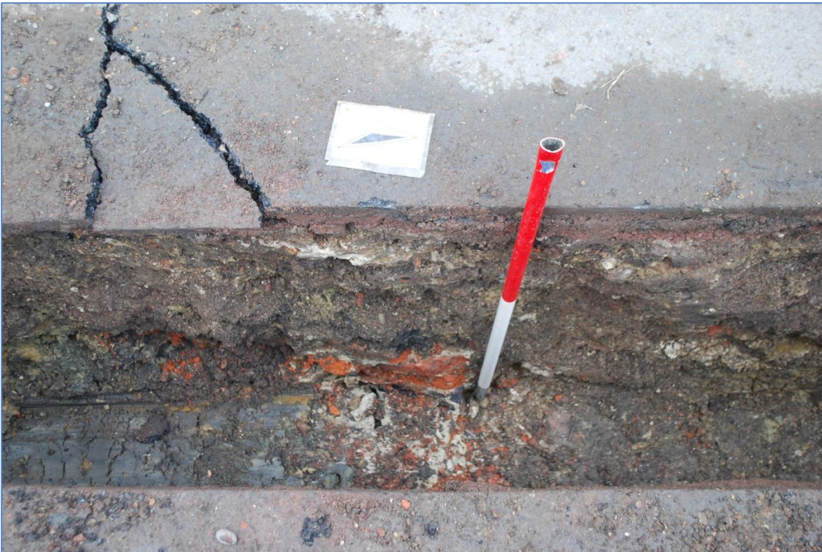
Plate 5 Brick wall footing in Trench 2 drainage replacement, previously cut by drain. View west.
