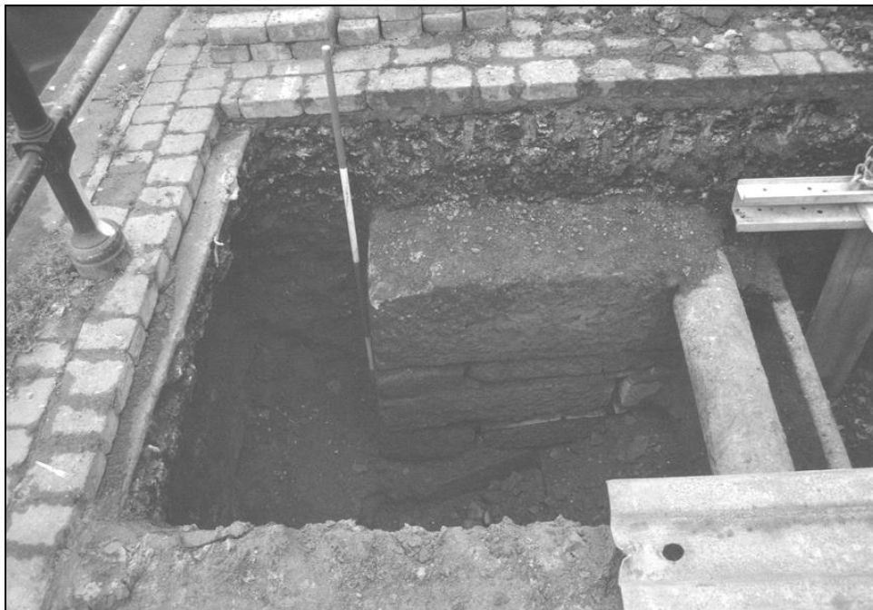
Plate 2: Break in former quayside wall exposed in test-pit 2
