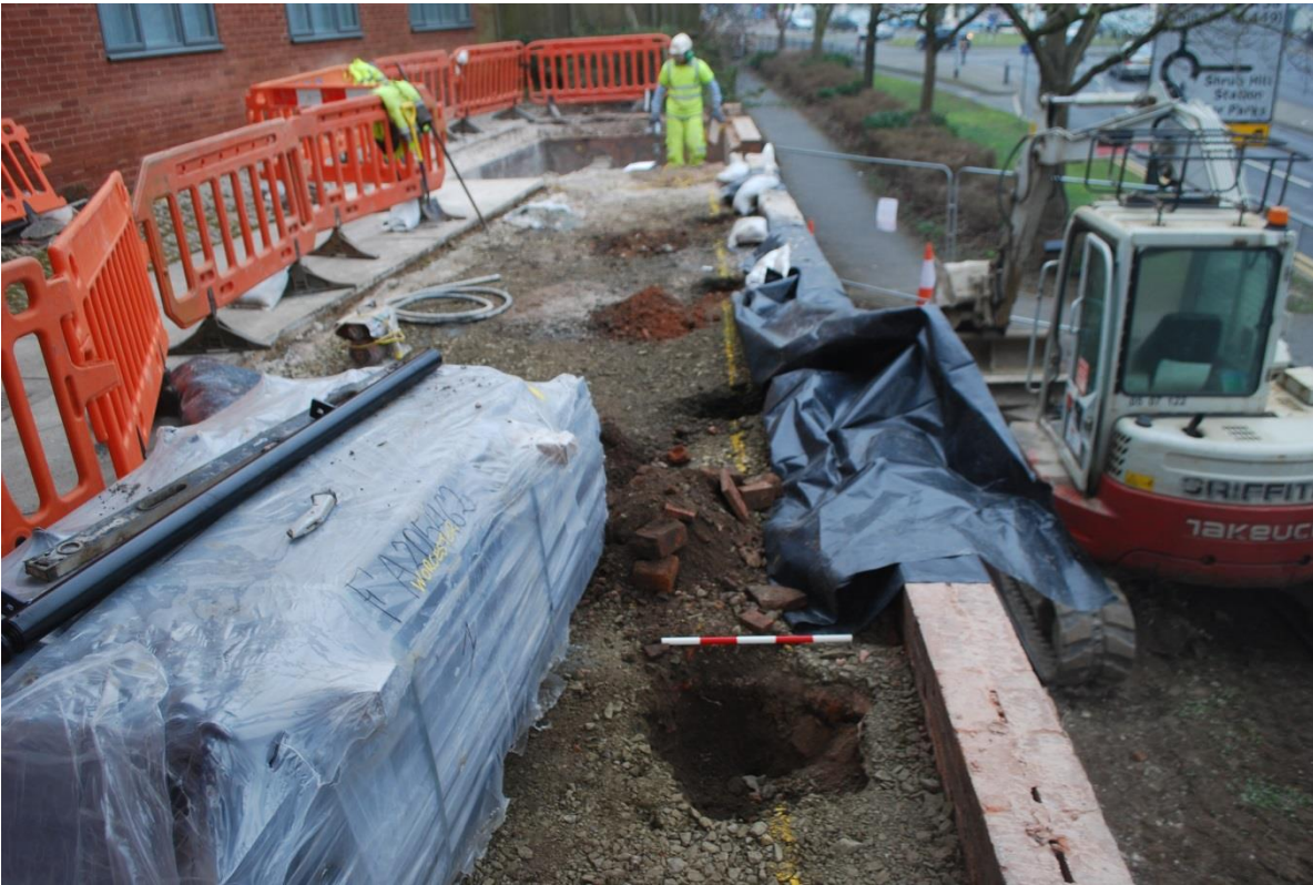
Plate 13: Fence posts 2 metres apart and 0.60m from face of wall after hand excavation
