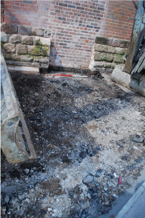
Plate 15: Tarmac removed from footpath to City wall access after blocking up. View northwest.
