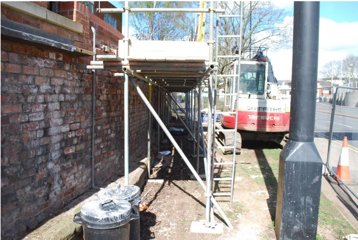
Plate 8: Scaffold for new brickwork. Not fixed to the Scheduled Monument City wall; View north
