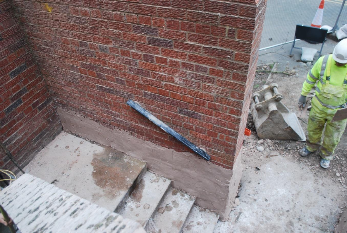
Plate 11: Sandstone wall covered by lime mortar fillet prior to concreting stairwell. View northwest
