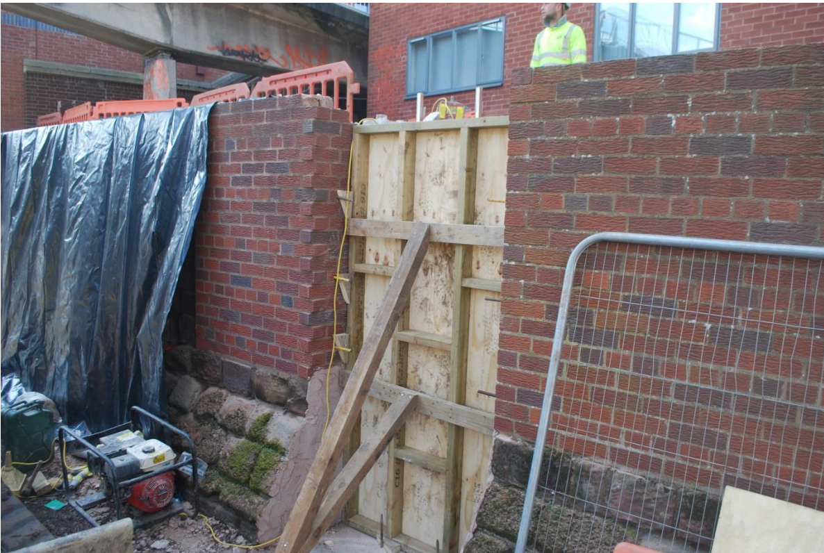
Plate 12: Stairwell shuttering and wall covered by plastic sheeting to protect from concrete.
