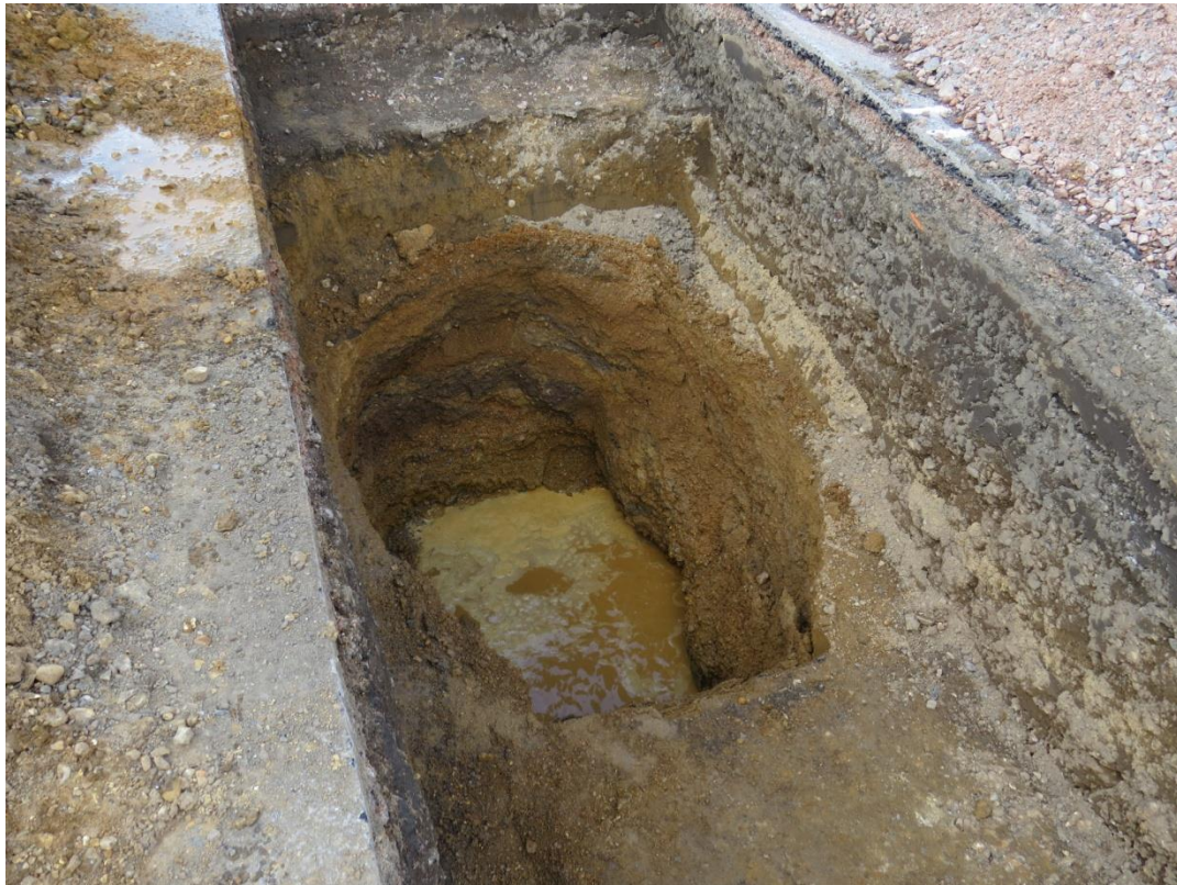
Plate 6. North and west faces of TP 6 showing stratigraphy of made ground and Pleistocene sands and gravels. Severe collapse and water penetration prevented exposure to bedrock.
