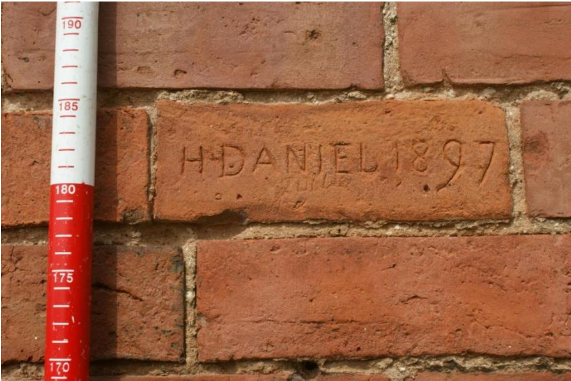
Plate 20 Graffiti on eastern gable, looking west
