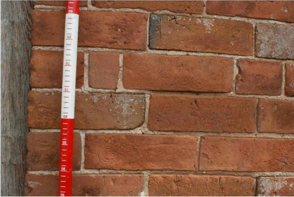
Plate 23 Graffiti by ground floor door, looking north
