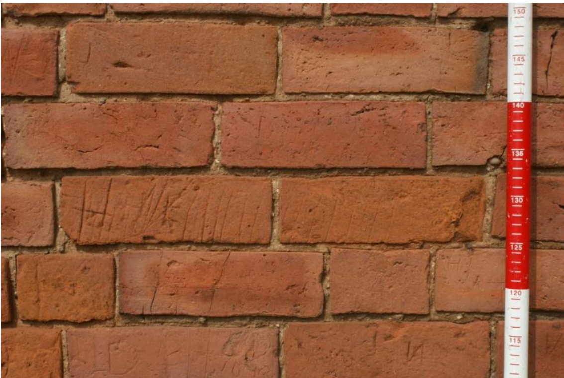
Plate 21 Graffiti on eastern gable, looking west
