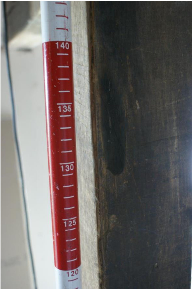
Plate 12 Candle burn mark on first floor truss, looking south-east
