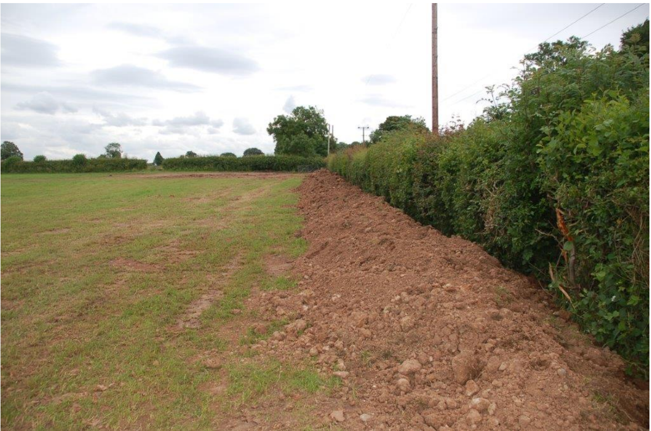
Plate 6 Backfilled drainage trench along southern boundary of site, completed prior to watching brief commencement, view south-east
