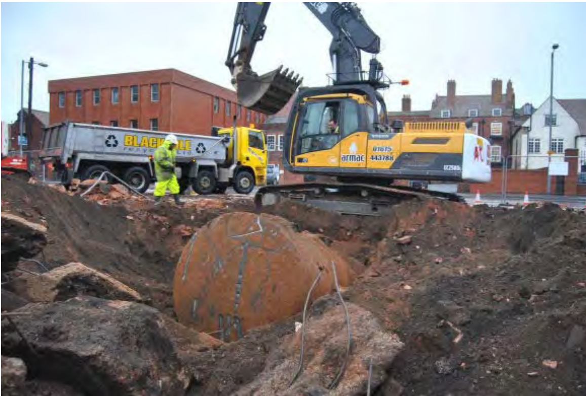
Plate 1 Removal of the fuel tanks during the watching brief from the west
