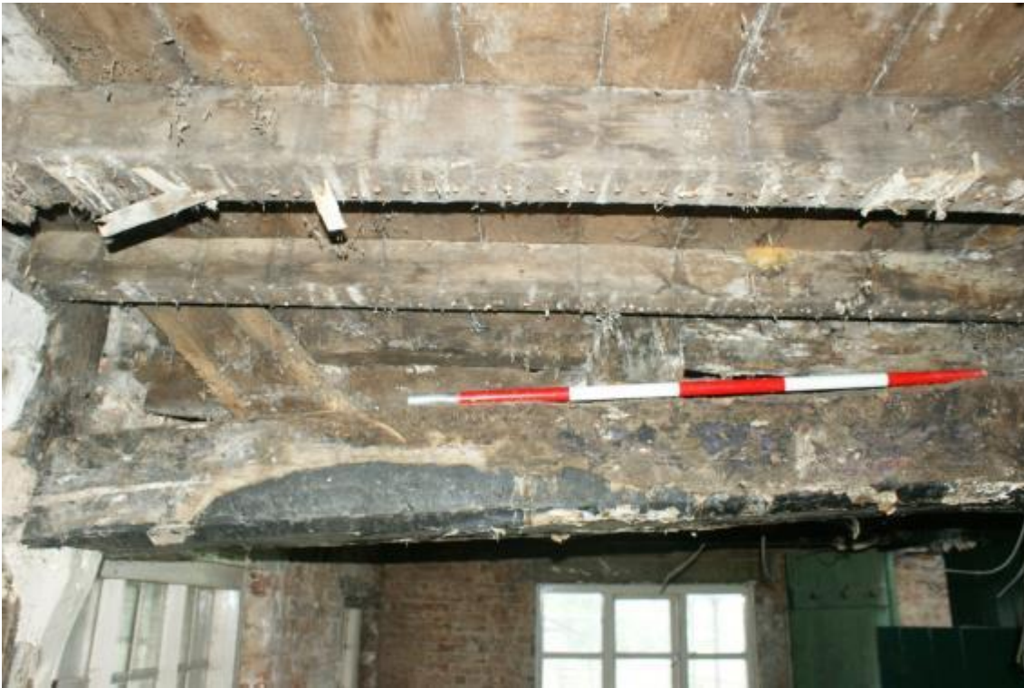
Plate 16 Phase 1 former gable framing visible above a north south aligned beam in the later kitchen, looking east.
