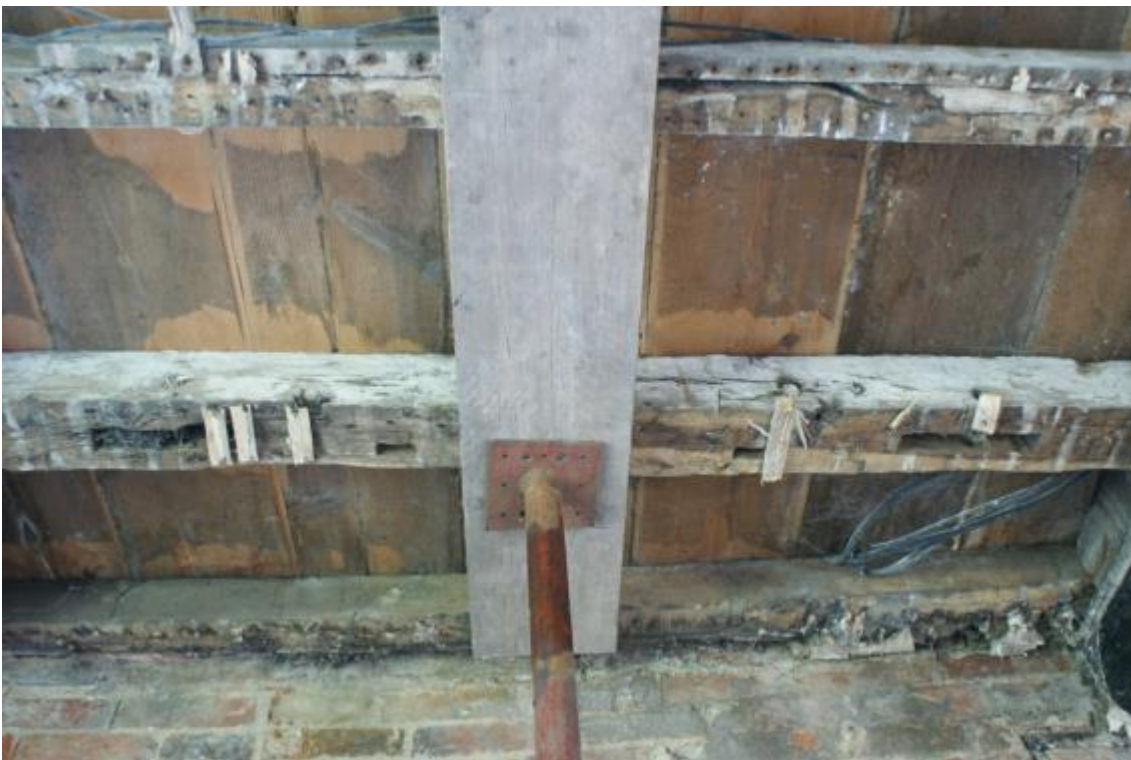
Plate 8 Timber reused as a Phase 4 floor joist showing evidence of window framing, looking north
