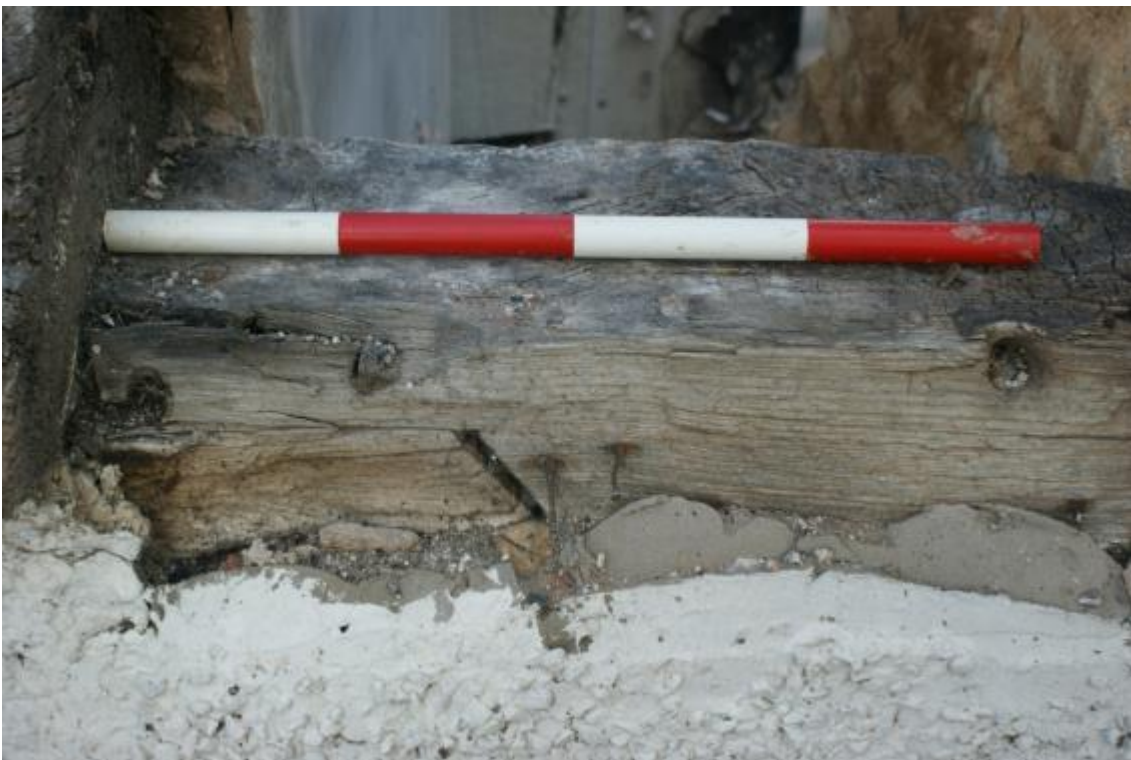
Plate 28 Phase 3 scarf joint in the wall plate to the east of the Phase 1 gable, looking north
