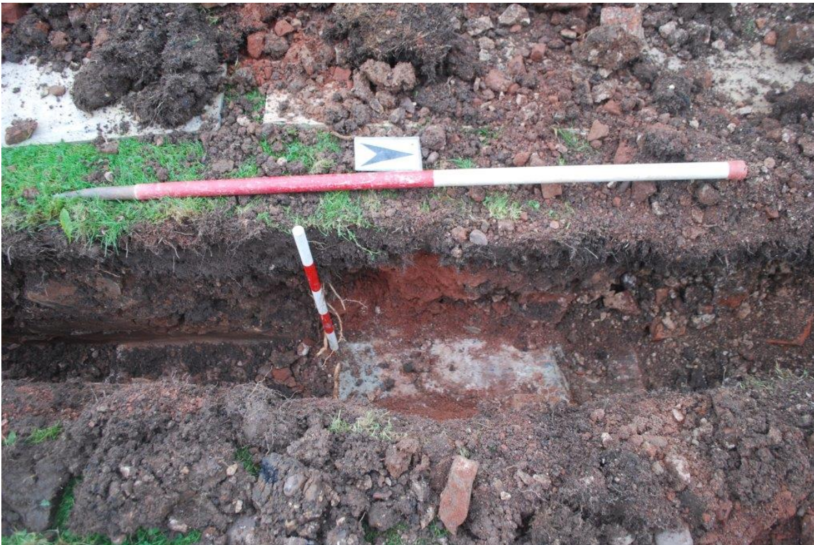
Plate 6 Sandstone wall footing 108, showing red sandstone upper and grey sandstone base, looking west
