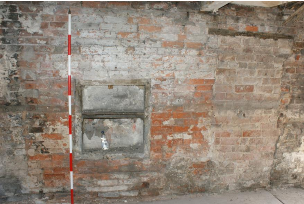
Plate 3 Blocked window in Phase 1 gable end, looking north-east
