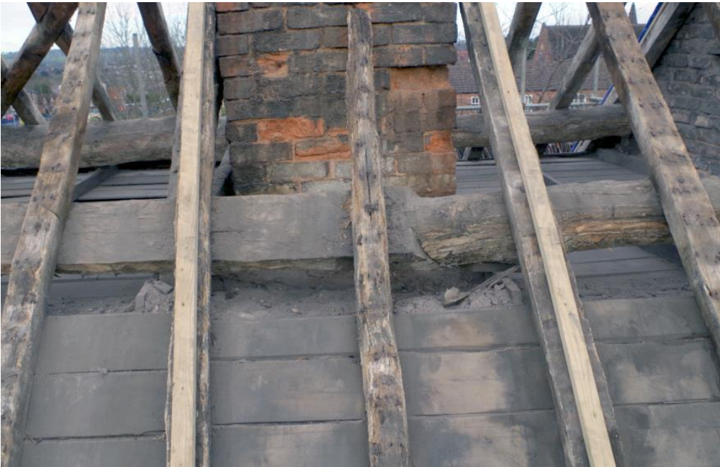
Plate 19 Phase 1 roof structure with scarf joint joining an extra section of purlin, looking north-west
