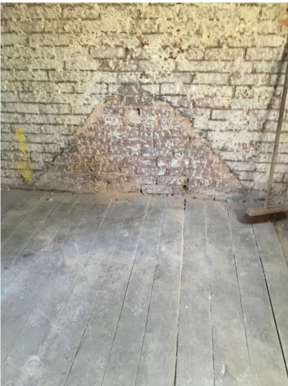
Plate 25 Evidence of the Phase 2 former roofline on the Phase 1 gable, looking north-east
