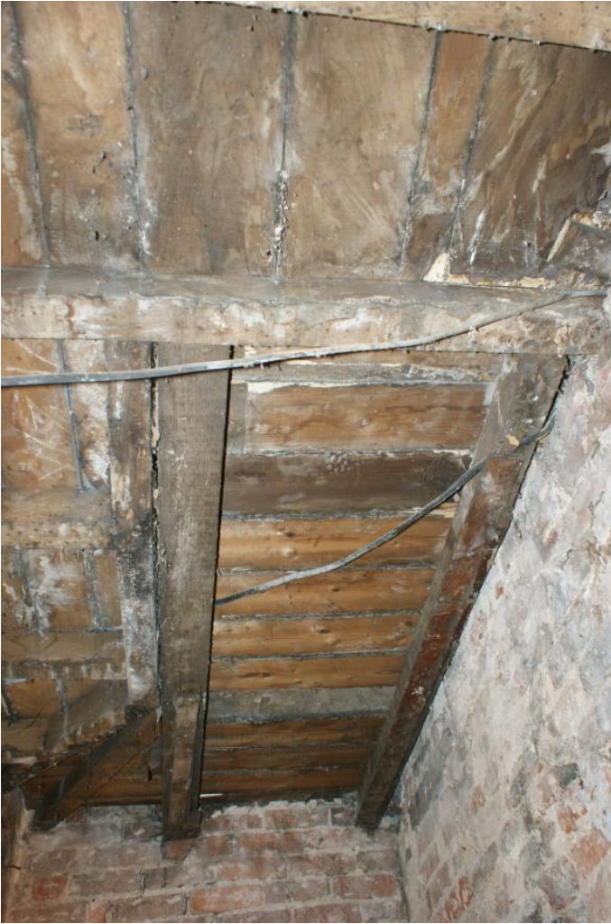
Plate 32 Phase 3, Number 21 ground floor showing evidence of former stairs position, looking south-west
