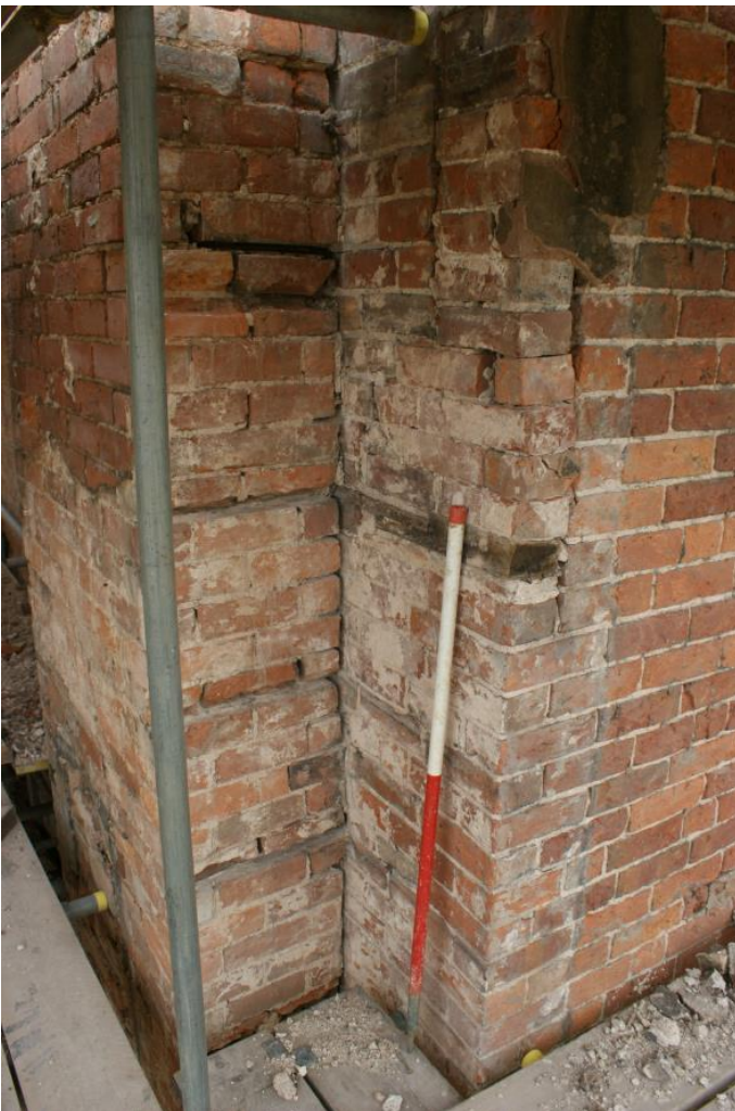
Plate 38 Phase 3 first floor former cupboards of the former Cock Inn, Number 20 gable, looking north
