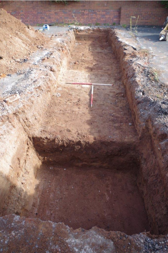
Plate 7 Trench 2 looking east showing sondage at west end of trench and natural gravel bands
