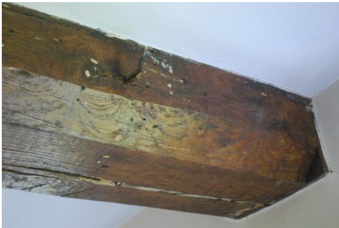
Plate 9 Phase 1 ground floor room with simple chamfer on the central beam, looking south-west
