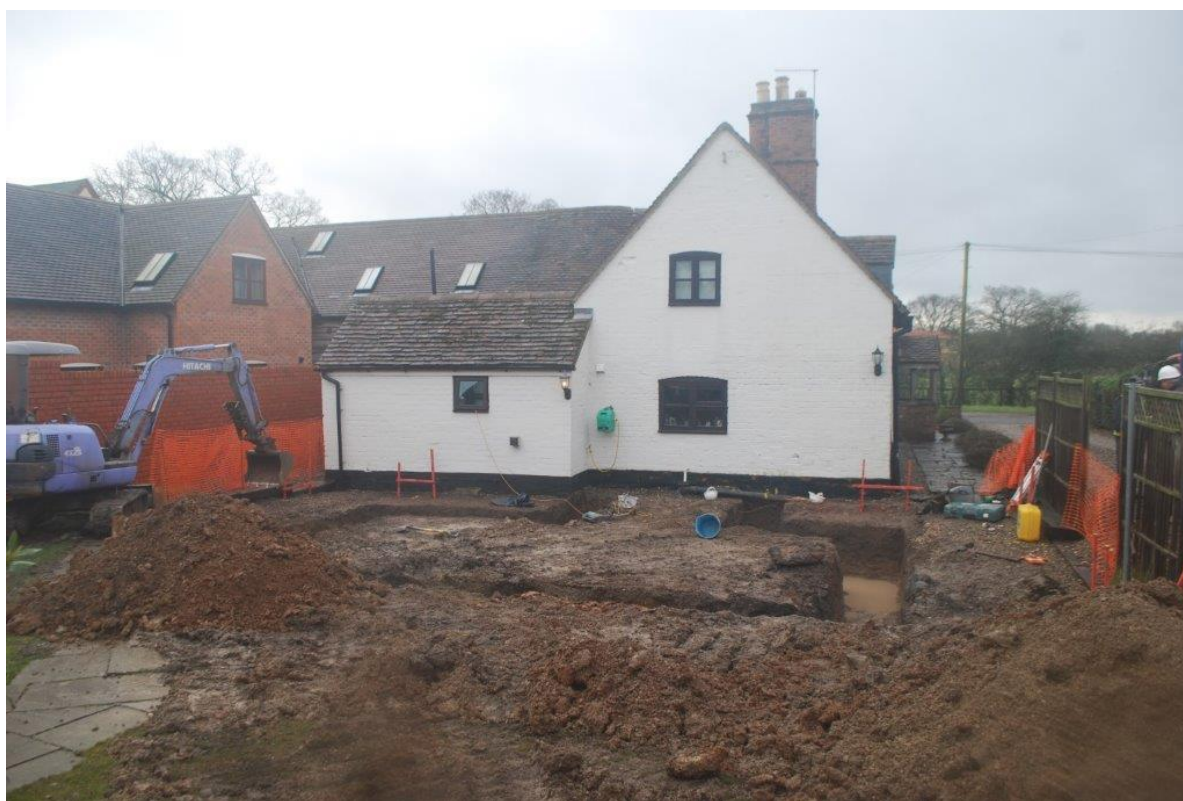
Plate 9 The rear of Brickwalls farmhouse following excavation of the foundations. View south.
