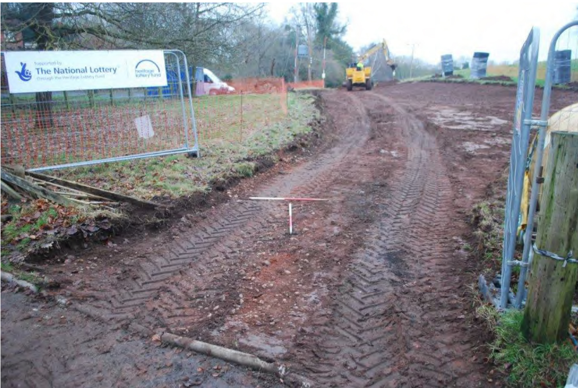
Plate 8 Entrance into car park stripped showing modern truncation of service trench backfill and made ground. View north. 2 x 1m scales.
