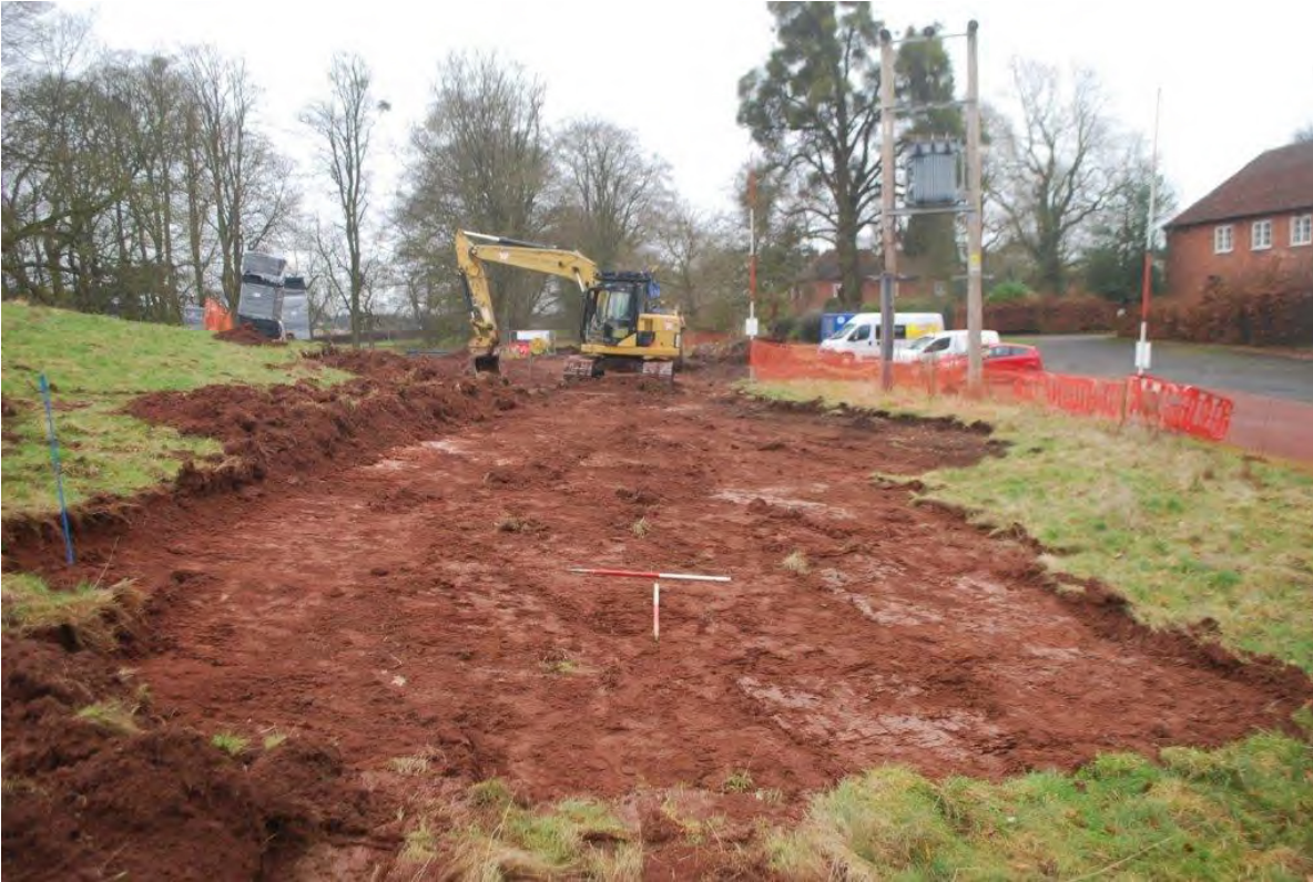
Plate 9 The northern part of the site onto solid sandstone geology and natural reddish orange clayey sand and marl. View south. 2 x 1m scales.
