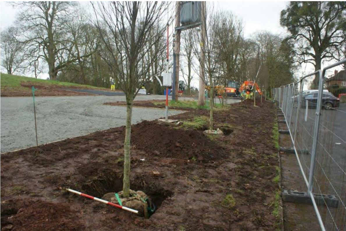
Plate 12 The tree pits following excavation from the north-west end of the site. View south-east. 0.5m scale.
