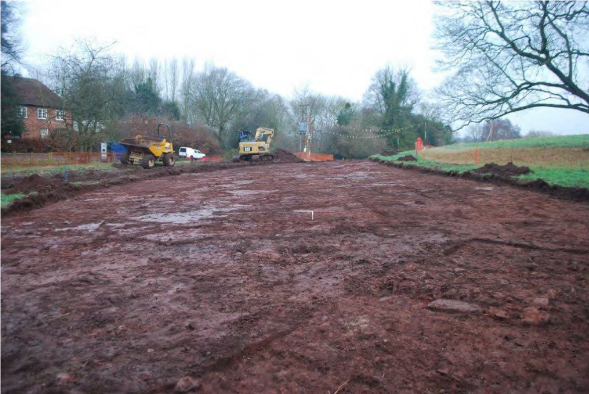
Plate 1 The car park stripped to subsoil depth. View north. 2 x 1m scales.
