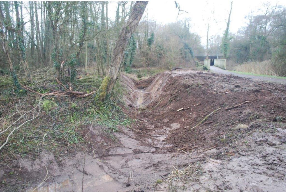
Plate 10: Re-profiled leat to west of Pike's pool; view south-west; no scales (beyond the scope of the formal watching brief)
