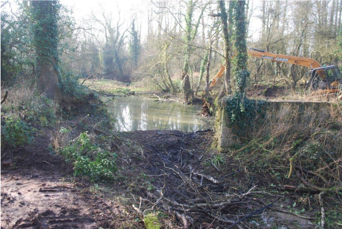
Plate 1 Pike's Pool prior to works de-silting the pond; view south; no scale
