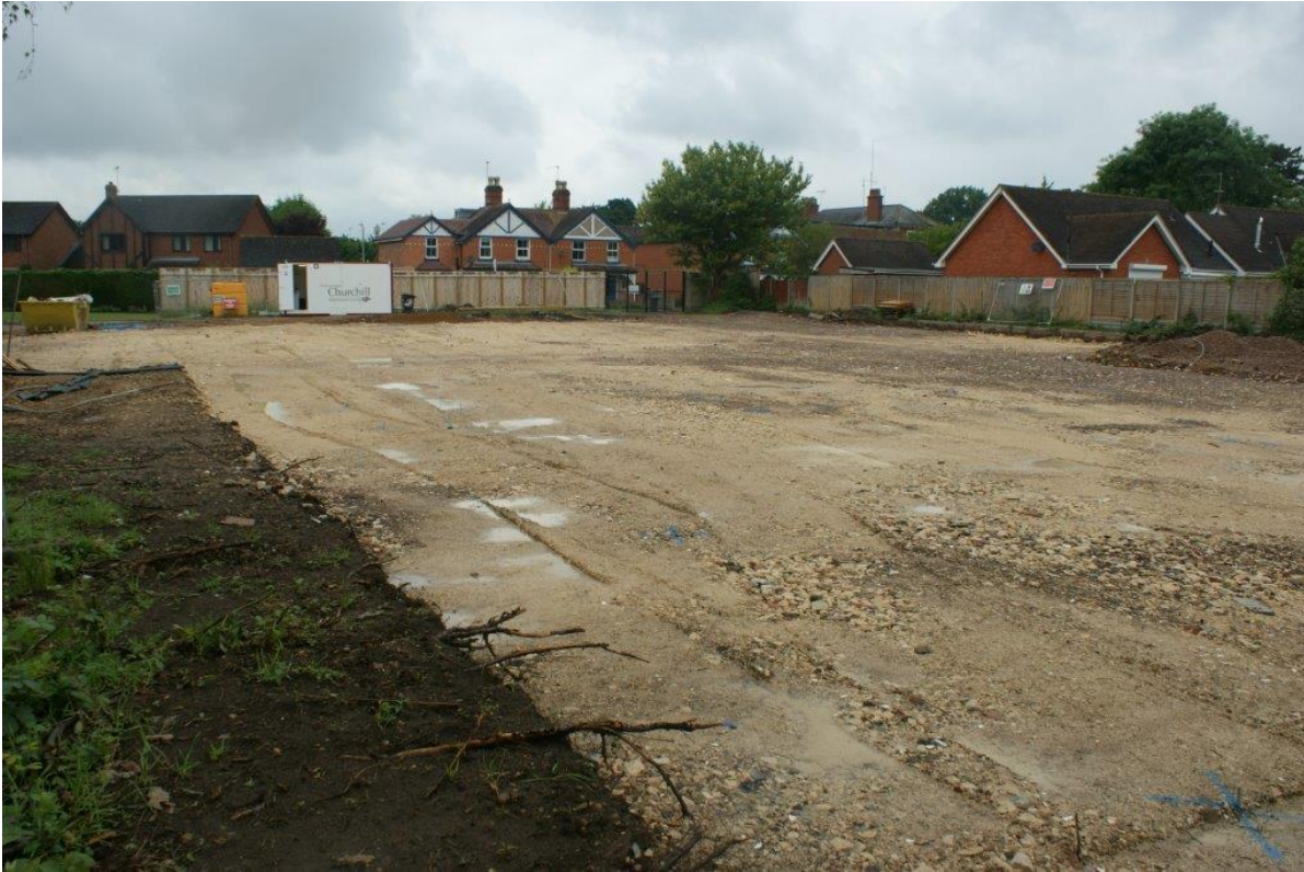
Plate 1 The site after demolition works, prior to groundworks, with a piling mat hardcore surface. View west
