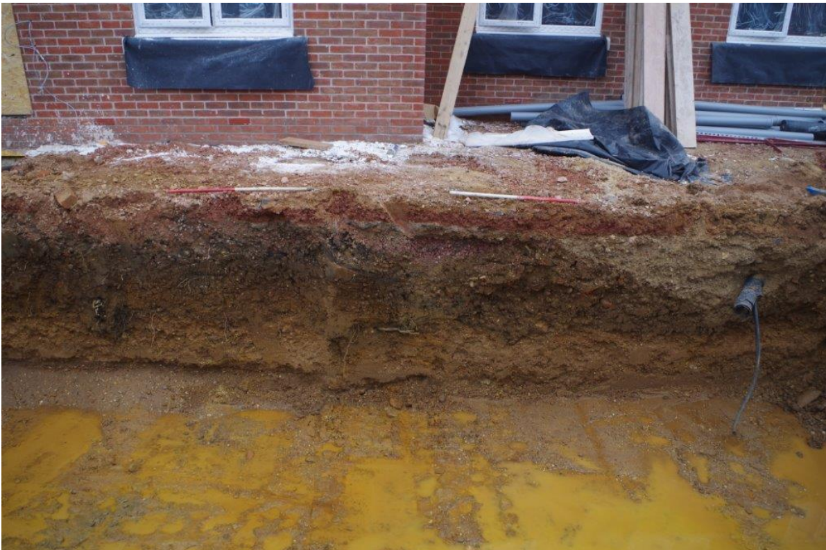
Plate 6 West facing section of Trench 3 attenuation tank showing general stratigraphy. 2 x 1m scales. View east
