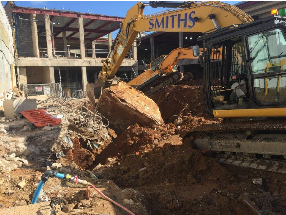
Plate 6: photograph illustrating the amount of concrete used to construct the Beechwood Arcade.
