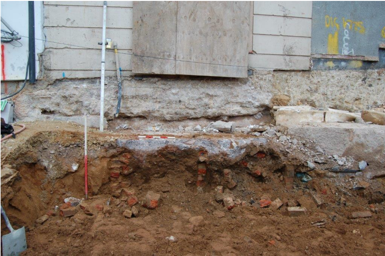
Plate 3: walls 300, 301 and 302 along the western boundary of the site. 1m and 0.5m scales
