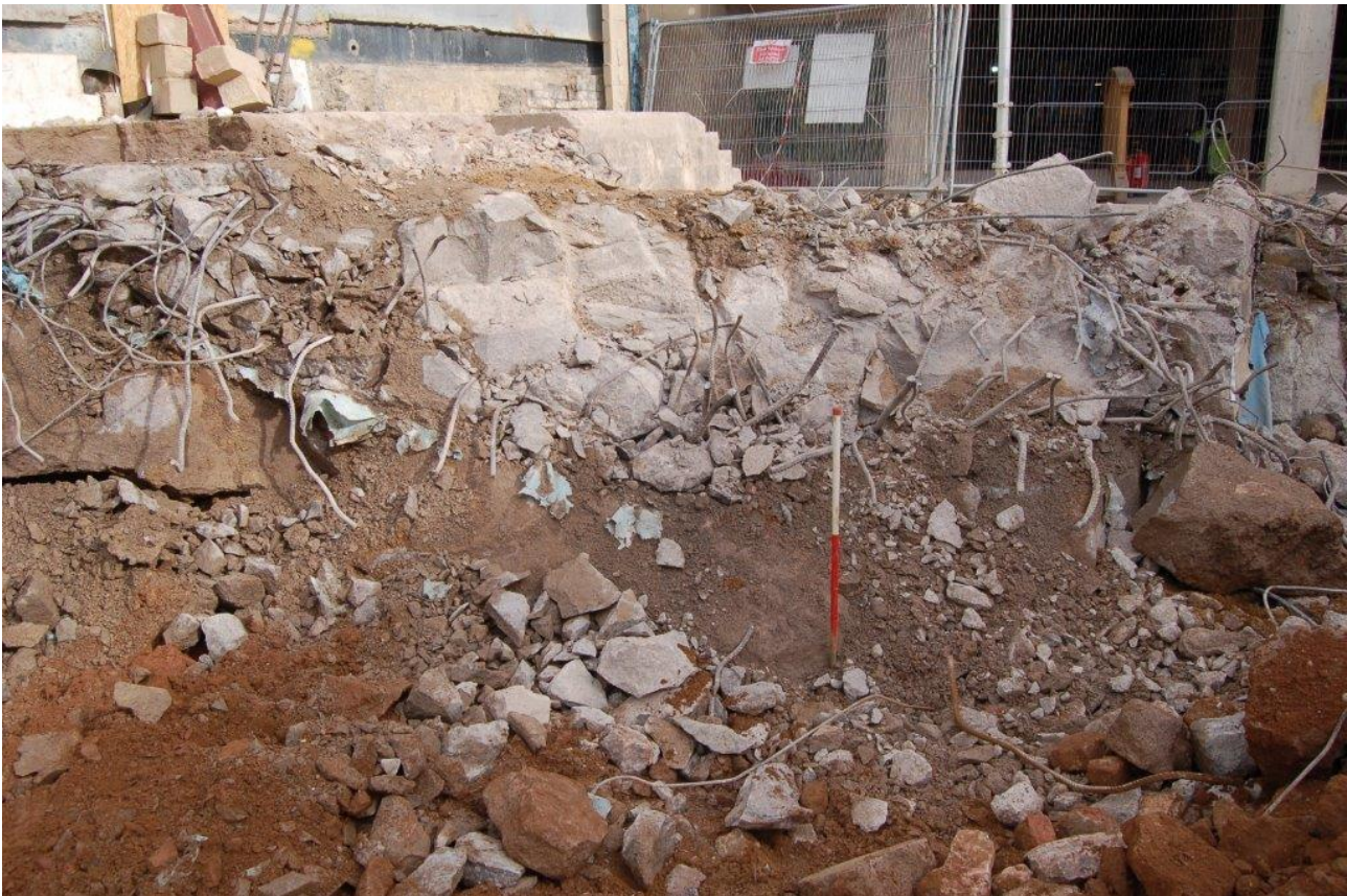
Plate 7: photograph illustrating the amount of concrete used to construct the Beechwood Arcade.
