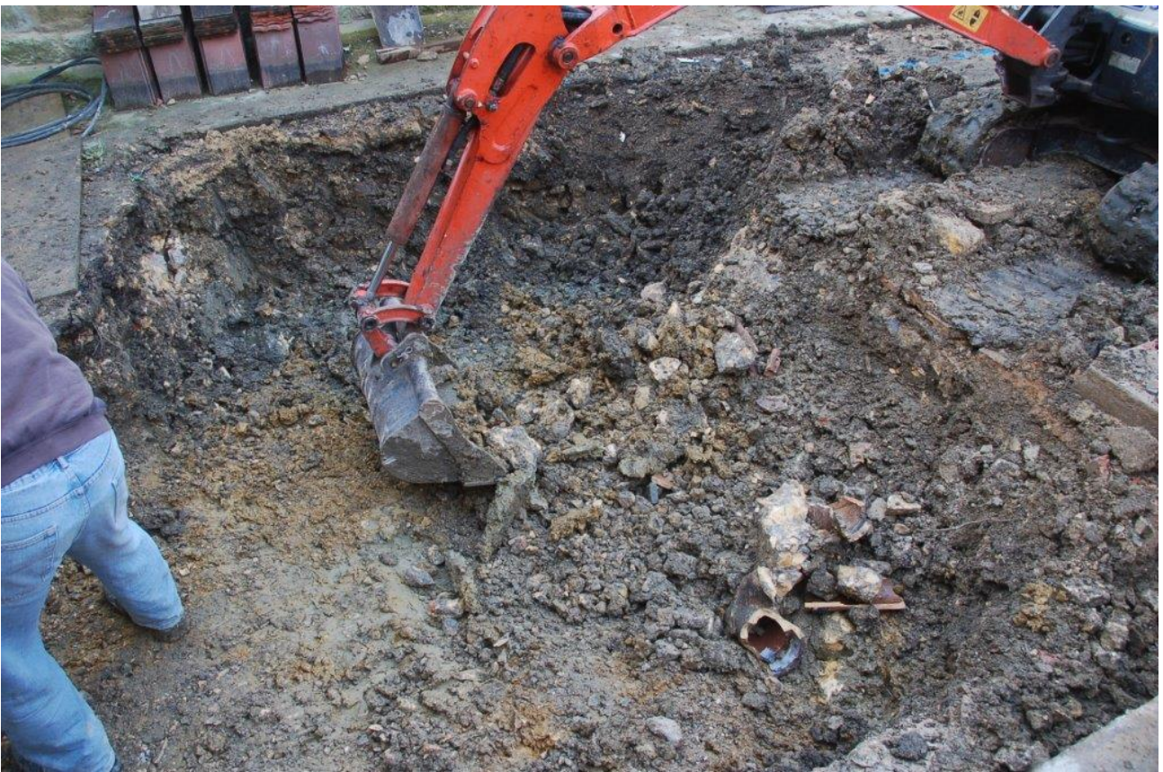
Plate 3 Working shot of machine excavation through deposits 104 and 101, view west, no scales
