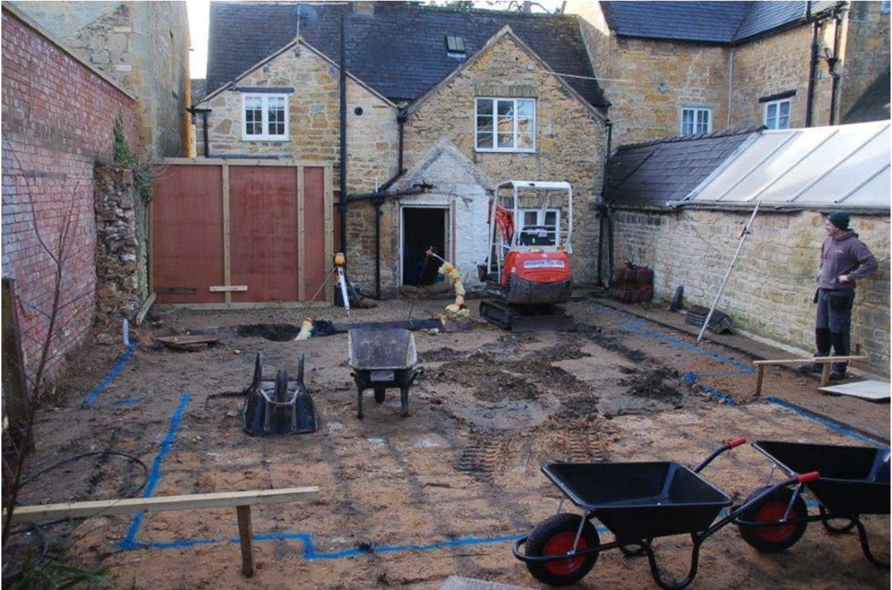
Plate 1 The site and trench layout, view south south-east towards property, no scales
